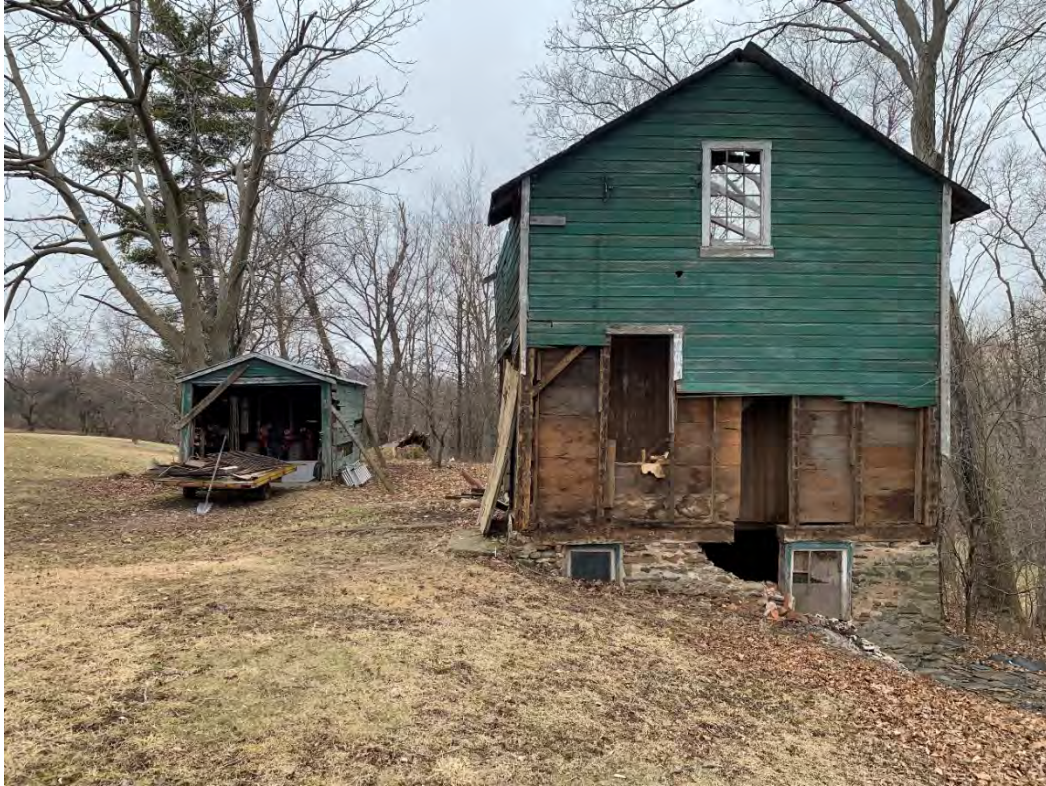
Figure 18: View of outbuildings along top of valley looking east towards North Service Line and Third Line (ML 2020).
