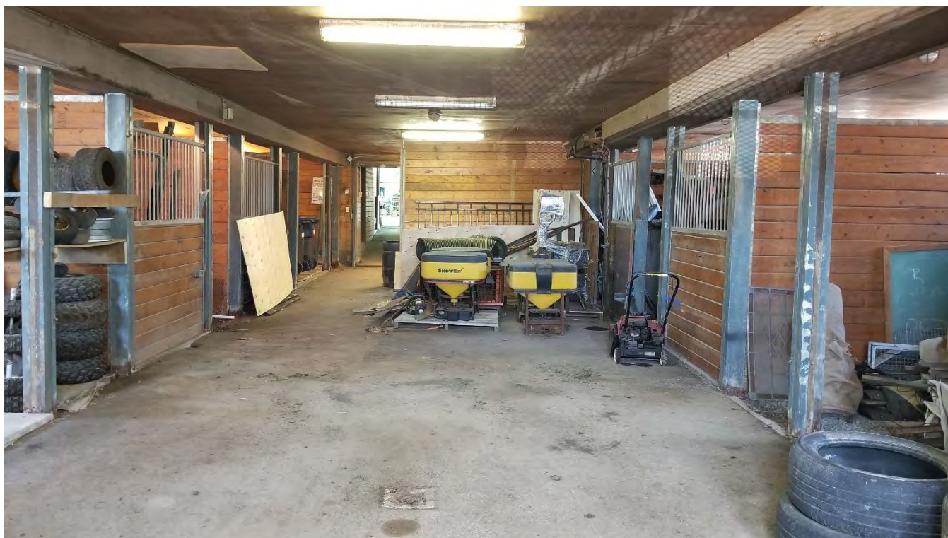
Figure 81 Central passage of the barn with stalls on either sides, looking northeast.
