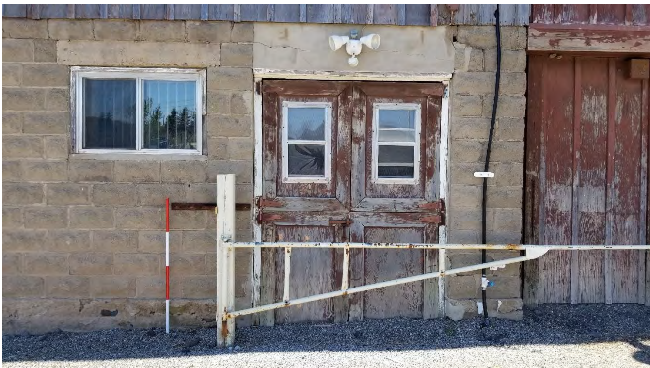
Figure 74 Double-leaf Dutch door in timber with one-over-one single hung windows and a concrete lintel on southeast elevation of the barn.
