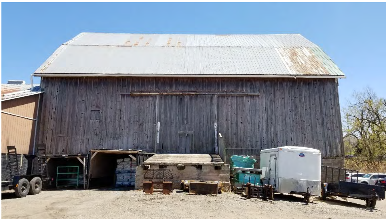
Figure 75 Partial wooden ramp and large central double sliding door on northwest elevation of the barn.
