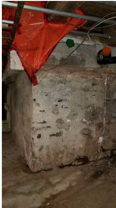
Figure 39 Basement looking north at raised foundation and opening to the left where the northwest foundation wall was cut and remove to join the basement of the rear extension.
