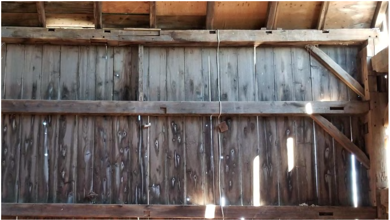
Figure 90 Posts, girts, and plate showing evidence of redundant mortices and treenail holes.
