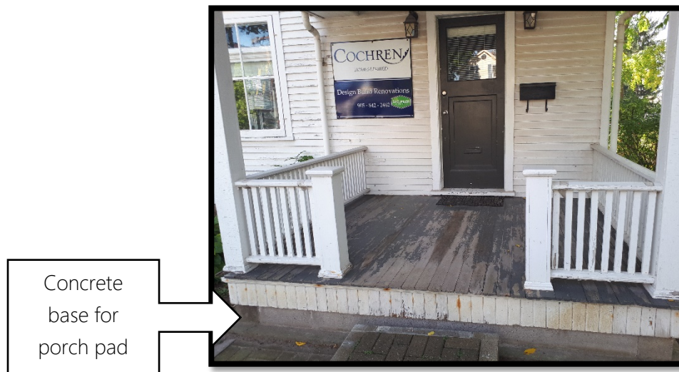
Figures 23 & 24: (Above) View of front façade showing condition of clapboard cladding, original windows and location where the front porch meets the façade; (Below) View of front porch with wooden handrail and columns and original door frame (MHBC, 2019)
