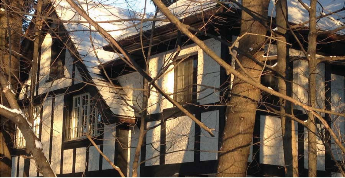
2.18 # 38 Second Street. The heavy texture and downward stroke used by the plasterer is similar to that at 320 Maple, but this former barn was heavily modified in the 1970's or later. The stucco finish has been installed on top of the cedar shakes on the steep roof. They are not more than 40 years old. While dramatic, this is a good example of a modern style of stucco that was not used in early 20 th century in Oakville.
