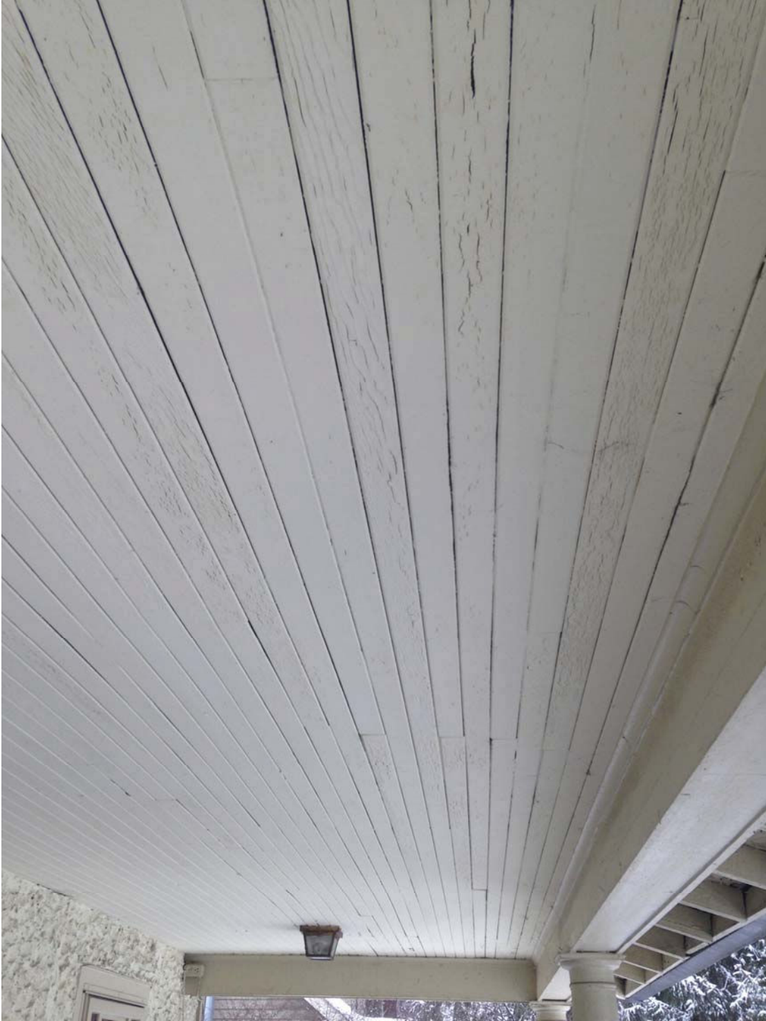
2.33 View of ceiling with visible shrinkage of the tongue and groove V-match material. Note the heavy checking in the paint which indicates that much of it will have to be removed to bare wood before repainting. The material was not kiln dried when installed. The stucco was applied up to the existing ceiling on the left side. Changes to replace the existing knob and tube connections in the ceiling would be best done from above by removing the roof, a pretty serious intervention.
