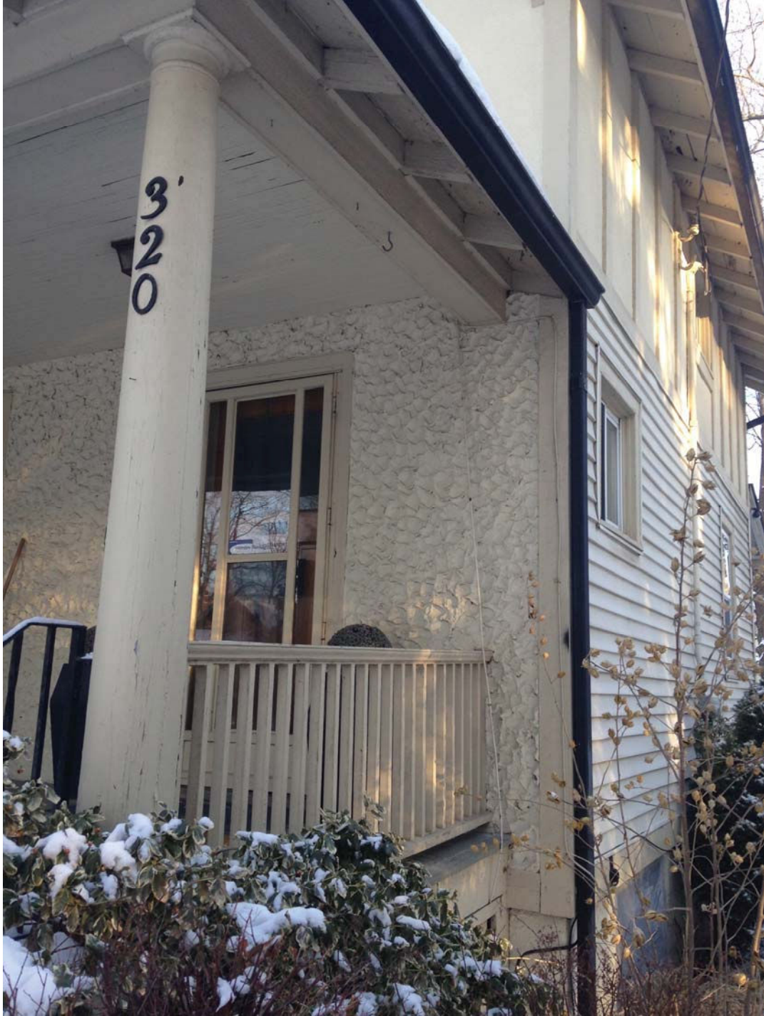
2.29 View of North West corner of verandah with vinyl siding, modern synthetic stucco and faux Tudor half-timber, concrete block foundation, and repaired stucco under the soffit. The Porch railing can be seen here, preceded the stucco. A wall cleat was installed to support the railing. This detail is often used where clapboard is installed after the railings, but also where stucco was applied up to the railing, so provides no conclusive proof that siding was or was not used originally.
