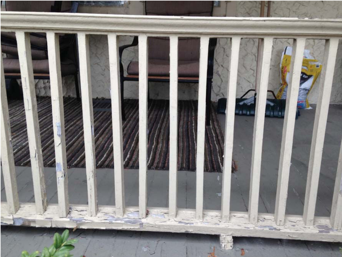
2.34 A “floating” rail with moulded hand and foot rails and square pickets was installed between columns. The foot rail is supported at mid span with blocks nailed to the deck to prevent sagging, and allow leaves to be swept clear. The crude blocking of the foot rail telegraphed the subsidence of the corners through the deck to the railing which has a bow of at least 2” along the front rail.
