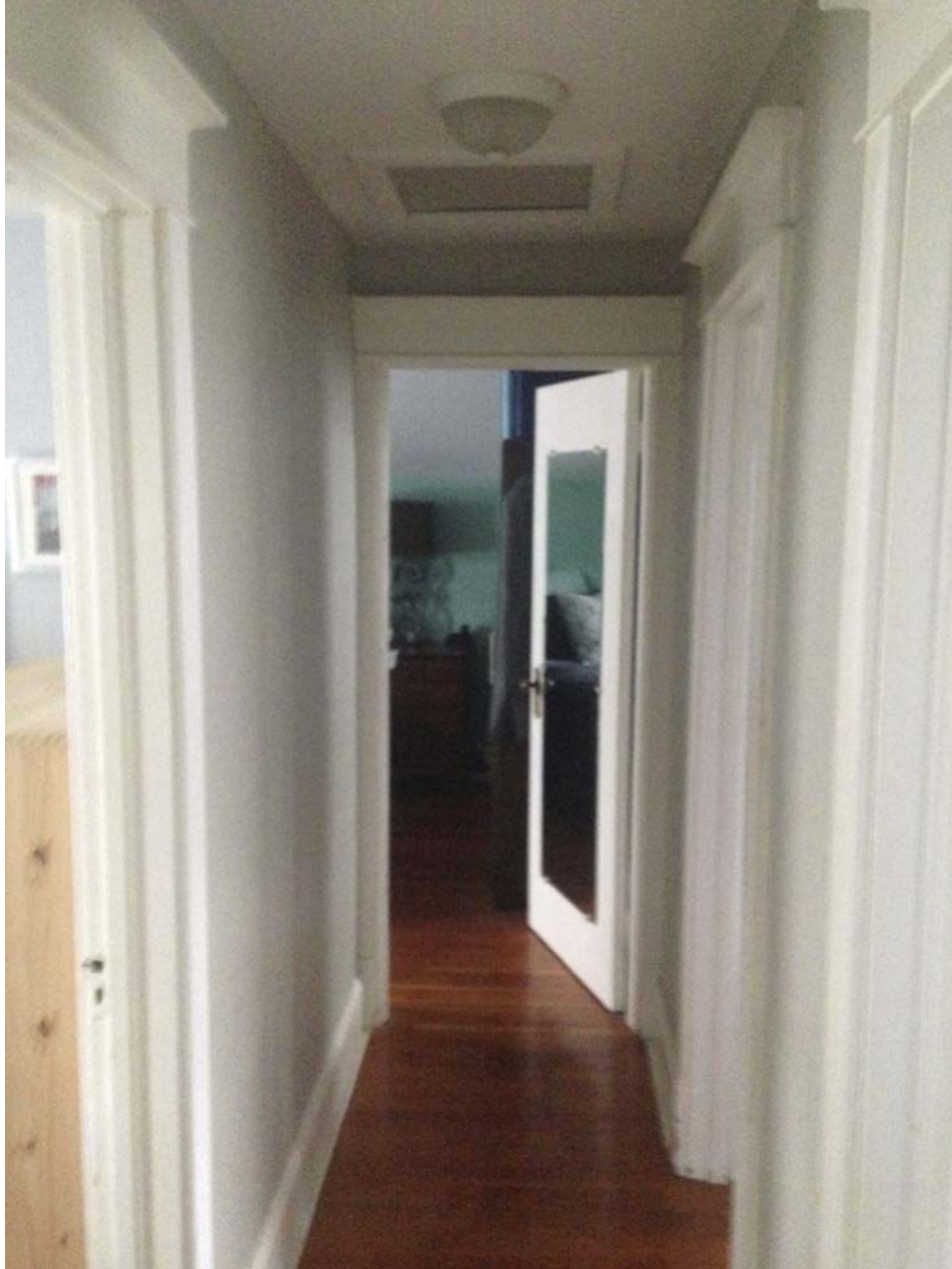
2.53 Second floor hallway is less than 36" wide. Attic hatch beyond light.
