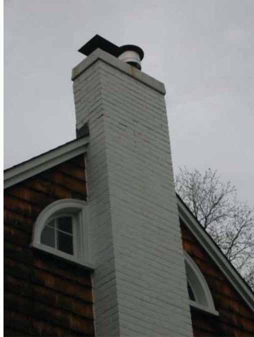
View of west gable end with white painted brick chimney and flanking quarter round windows
