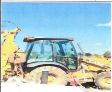
Pic 26- Road Blockage for construction of stacked town homes - by Biddington
