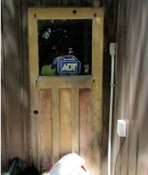
103. Door with paint peeling (South elevation)
