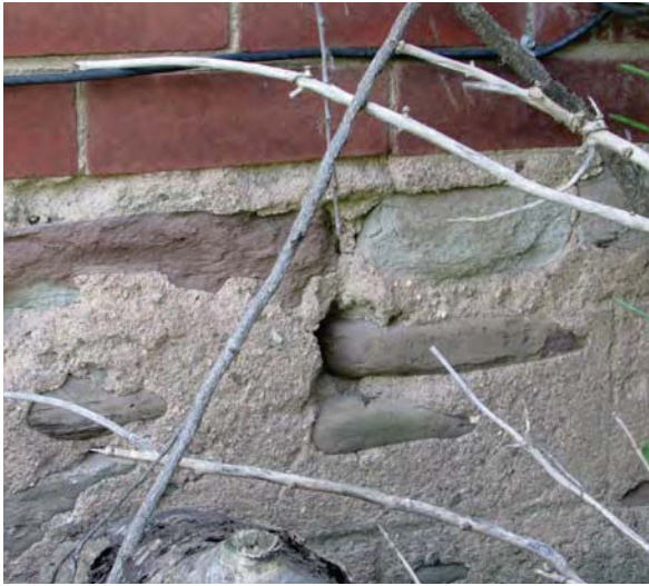
39. Deteriorated parging at base (North elevation)
