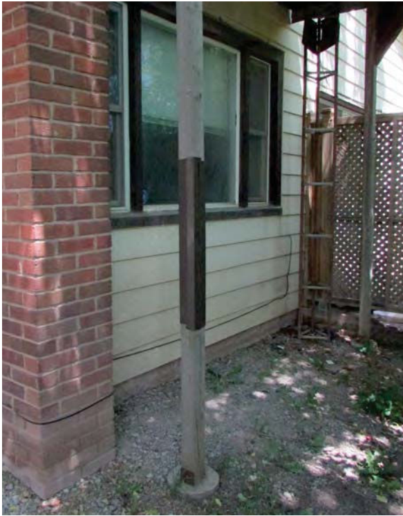
73. Metal support for timber post to deck above
