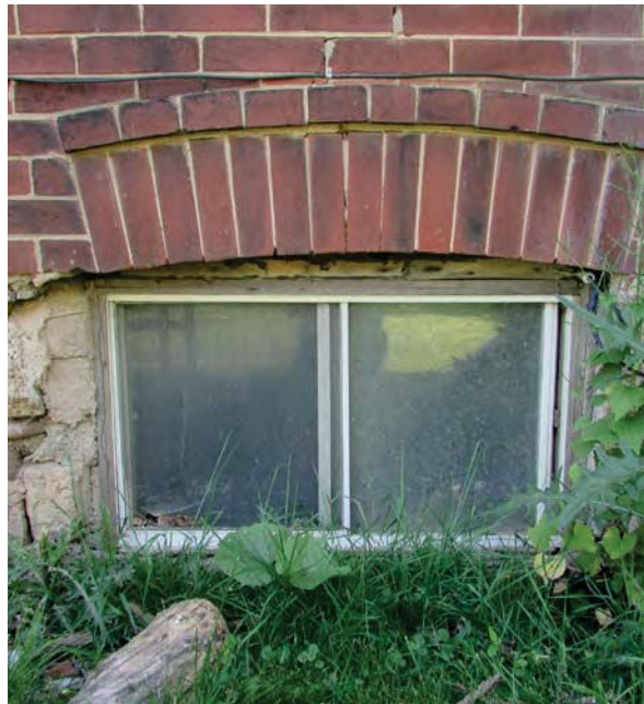
42. Poor condition of timber framed window (North elevation)
