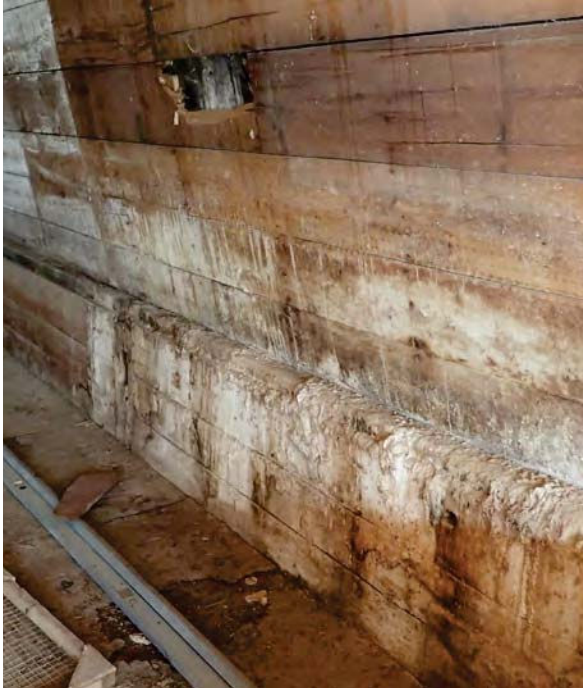
127. Excrement staining to wood wall planks, and hole in planks.
