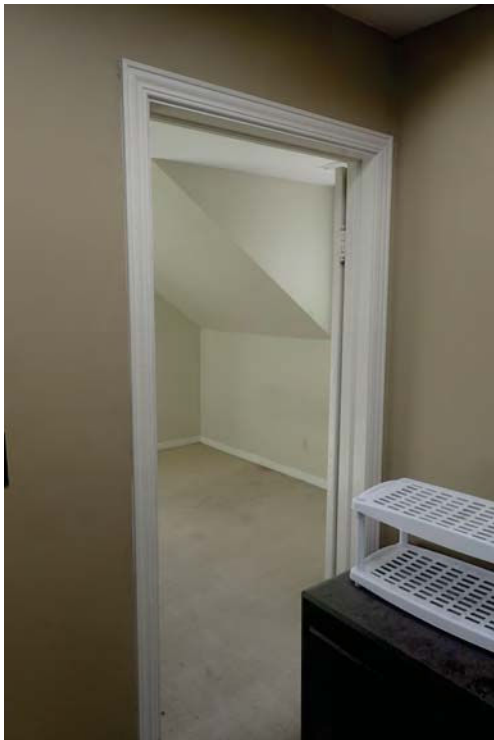
82. Good condition of walls and ceiling in 1860s section of the house.
