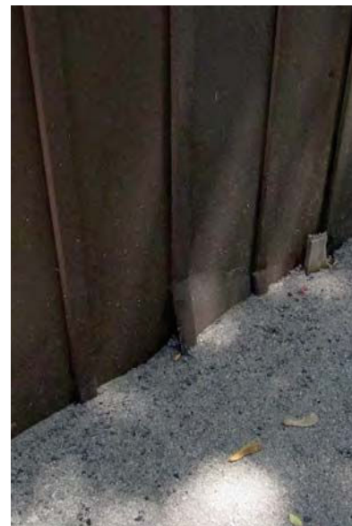
96. Dent to base of cladding (West elevation)
