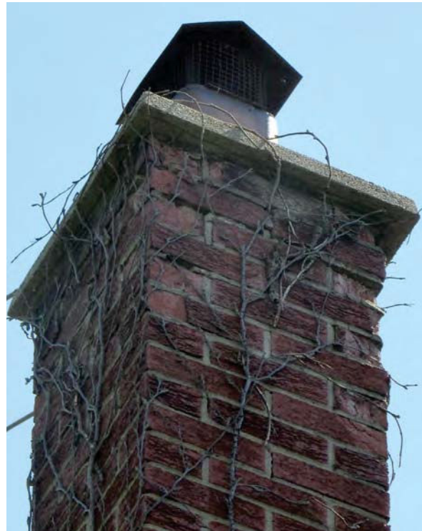
38. Spalled bricks and deteriorated mortar joints on chimney
