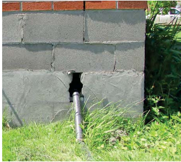
40. Hole in parging (East elevation)
