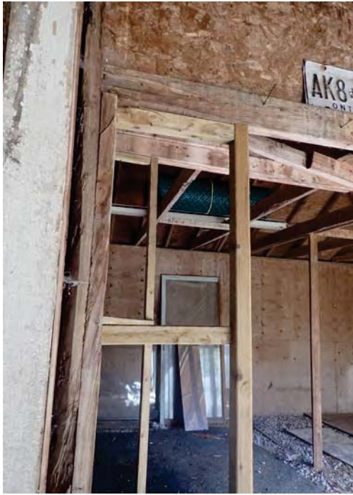
115. Fair condition of framing in Southern extension.
