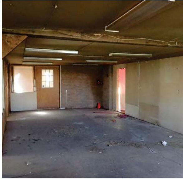
112. Fair condition of central section of first floor, looking towards West extension.
