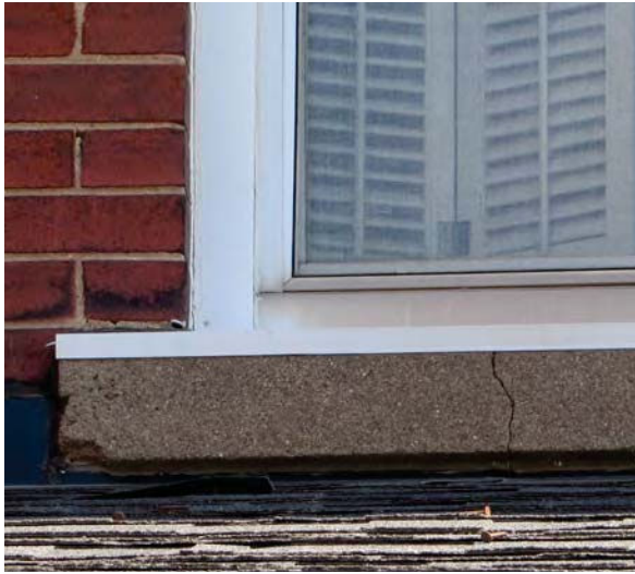
43. Crack and chip in concrete sill (West elevation).
