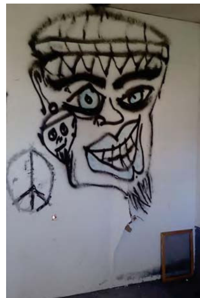
110. Graffiti, and damage to wall in Northern extension.
