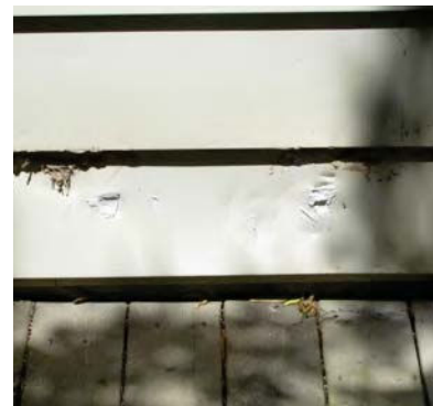
64. Dents to base of cladding (South elevation)
