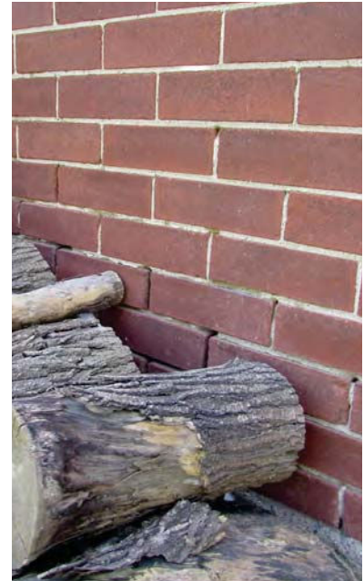
33. Deteriorated and open mortar joints (North elevation)
