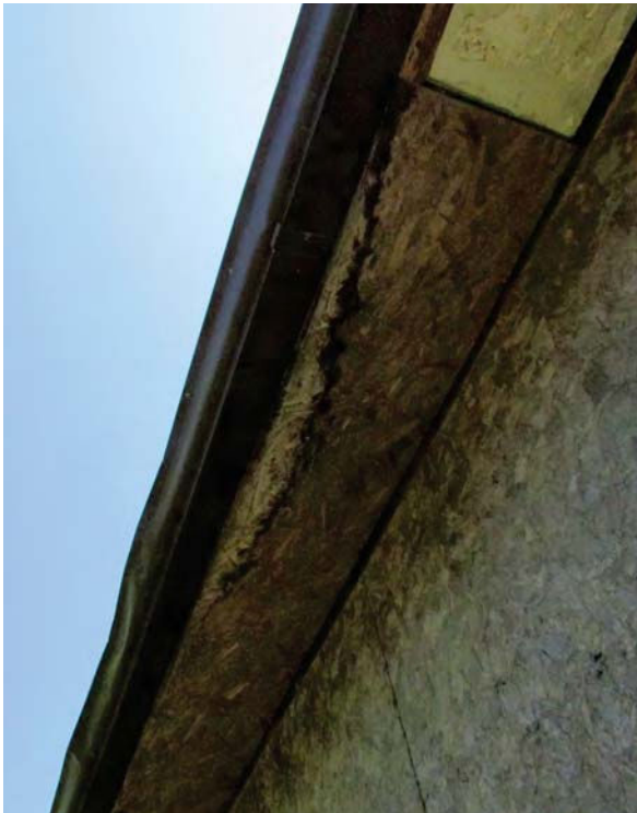
107. Missing soffit. Note water damage to particle board (North elevation)
