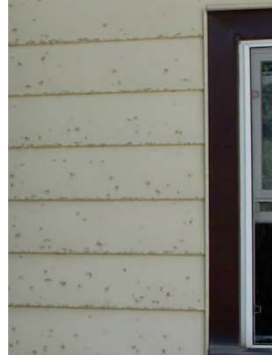
63. Chips to paint on metal cladding (North elevation)
