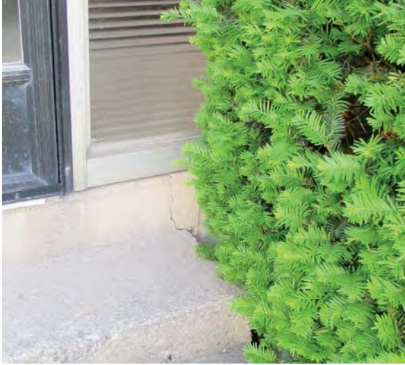
47. Crack in parking at base of porch (West elevation)
