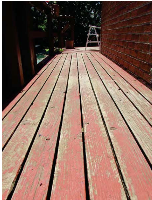
46. Poor condition of timber deck.
