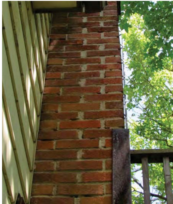
68. Increase in vertical mortar width as chimney height increases
