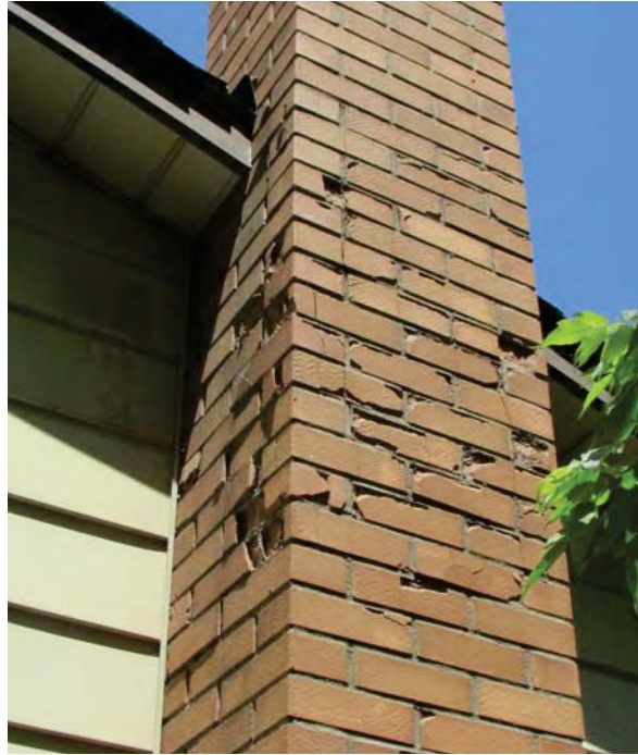
66. Spalled bricks at chimney
