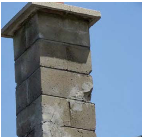
99. Chipped brick on chimney
