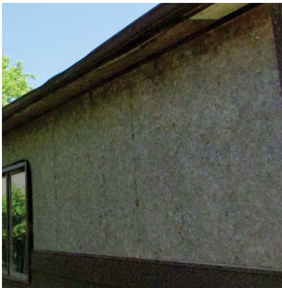
97. Missing metal cladding. Note dark stains at top of board indicating water damage (North elevation)
