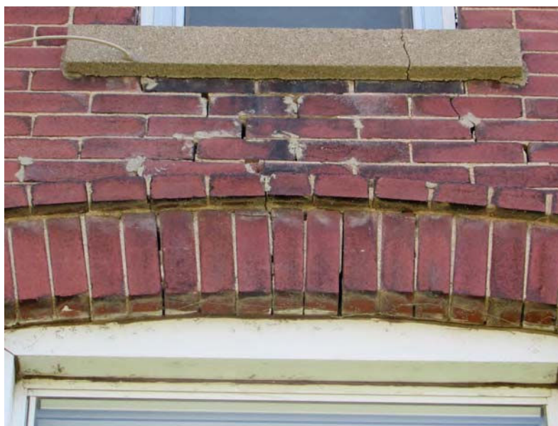
34. Stepped cracks between arch and sill, and deteriorated mortar joints
