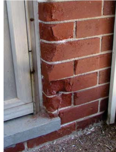
31. Spalled and chipped bricks at entrance (South elevation)
