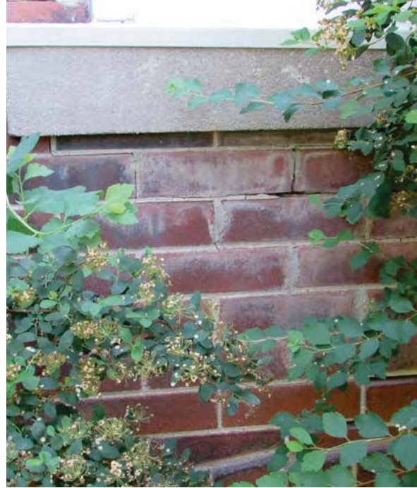
36. Stained bricks, and efflorescence under sill (West elevation)
