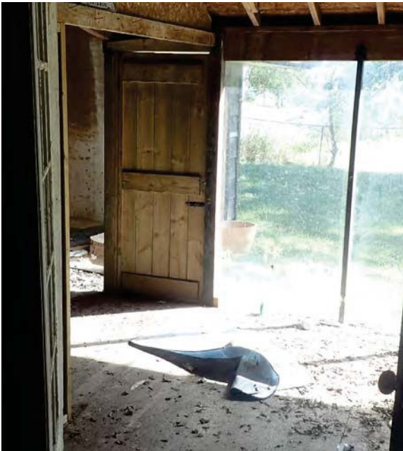
113. Poor condition of Southern extension.
