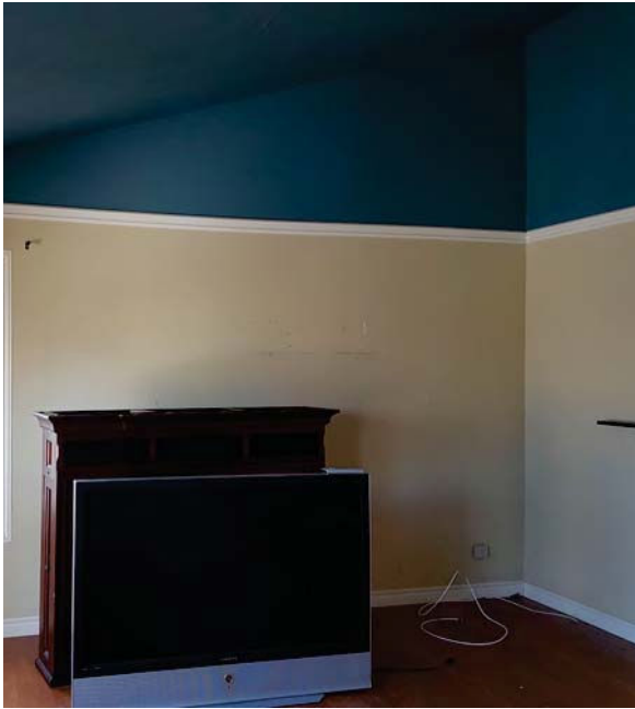
76. Fair condition of walls and ceiling in 1980s extension.
