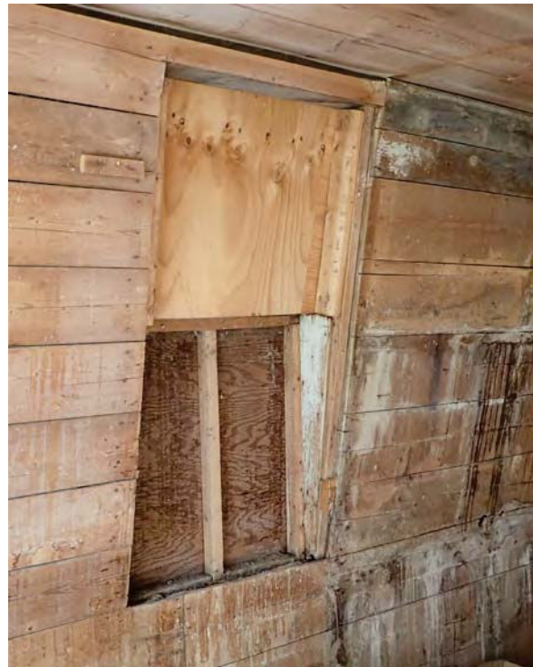
126. Boarded up window opening on second floor.
