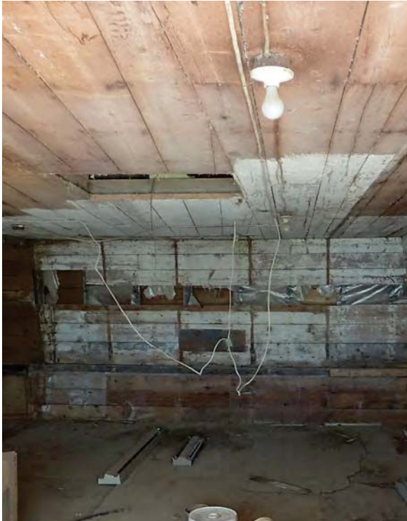
125. General condition of second floor, with missing planks of wood on wall.
