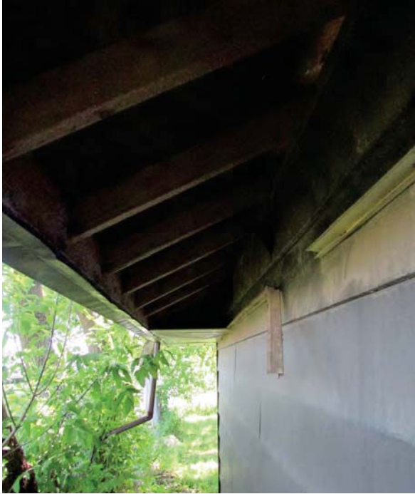
105. Missing soffit (Rear elevation)
