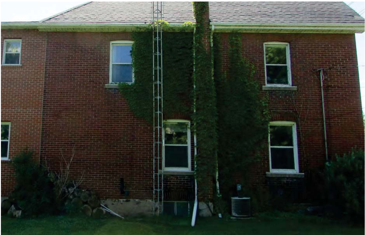
48. Vegetation on brick (North elevation)
