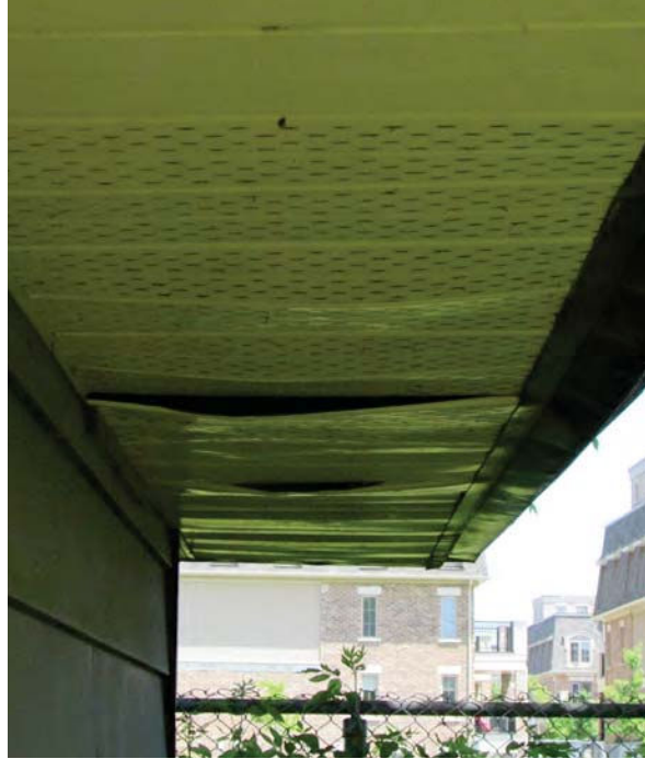
106. Damaged soffit (South elevation)
