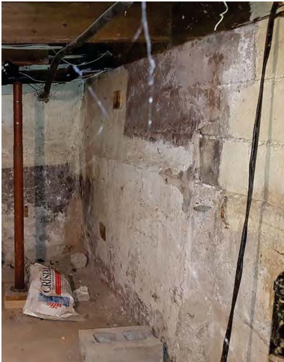
90. Cast concrete and concrete block walls in basement underneath 1860s section of the house.
