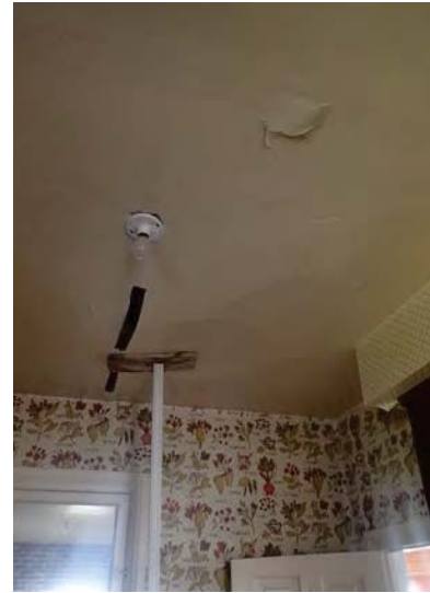
49. Cracked and damaged kitchen ceiling with temporary support.
