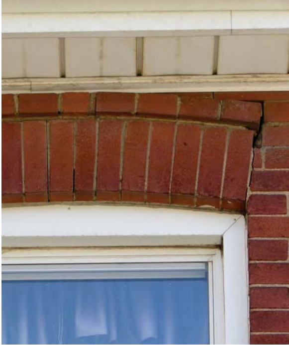
35. Deteriorated and open mortar joints (West Elevation)
