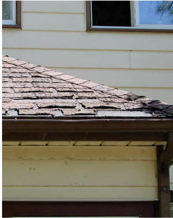
72. Deteriorated shingles on roof.
