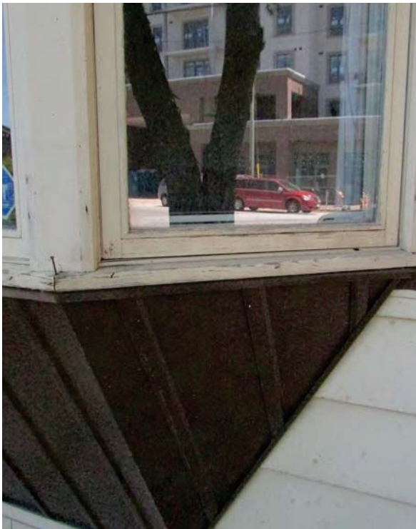
71. Weathered timber sill and frame at bay window (North elevation)
