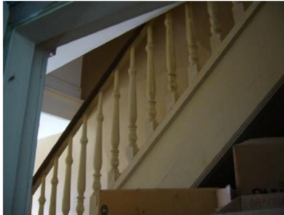
Interior of north office portion (136 Dunn Street) looking upwards to staircase to apartment at 134 Dunn Street, April 10, 2017
