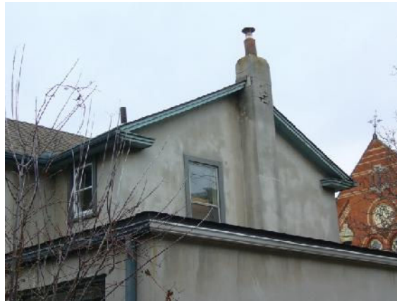
South façade with eaves return at roof level and altered windows, January 18, 2017.
