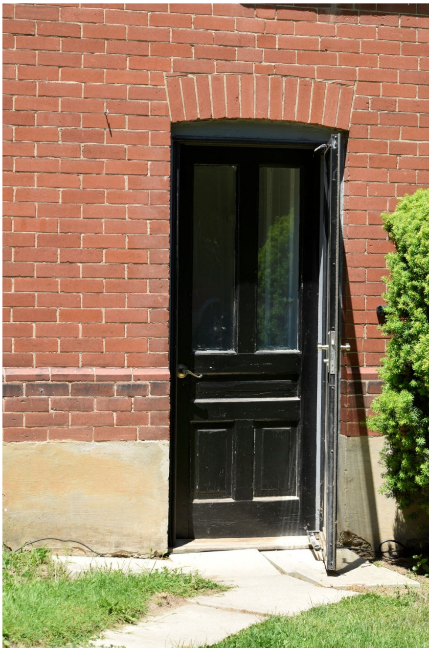
Image 10: Original frame and panel door with glass on south face, note jack arch and 45° beveled brick plinth cap
