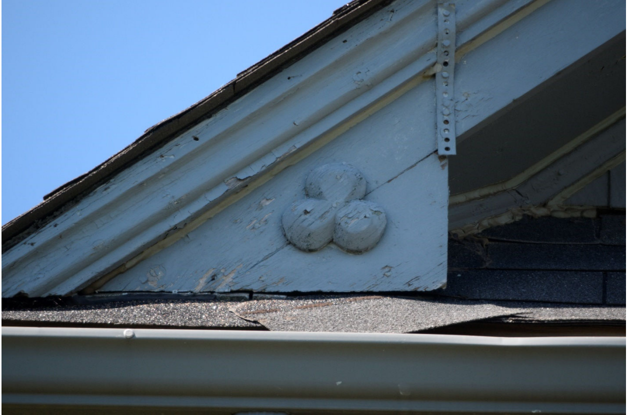
Image 9: Decorative trefoil detail on closed pedimented gable end, signs of water infiltration and evidence of attempted repair
