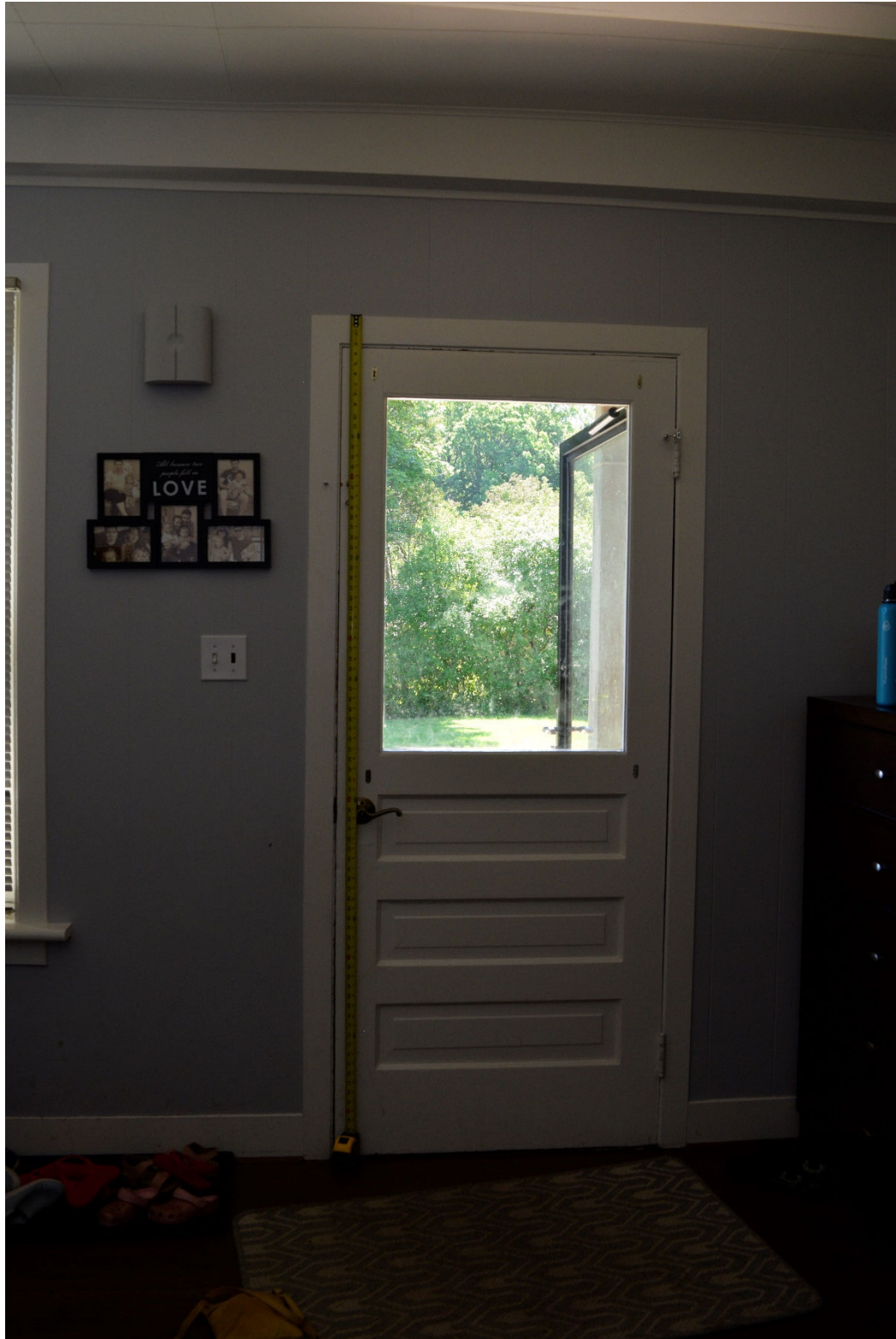
Image 22: Original frame and panel wood door on south face of residence, note non-original trim and baseboard
