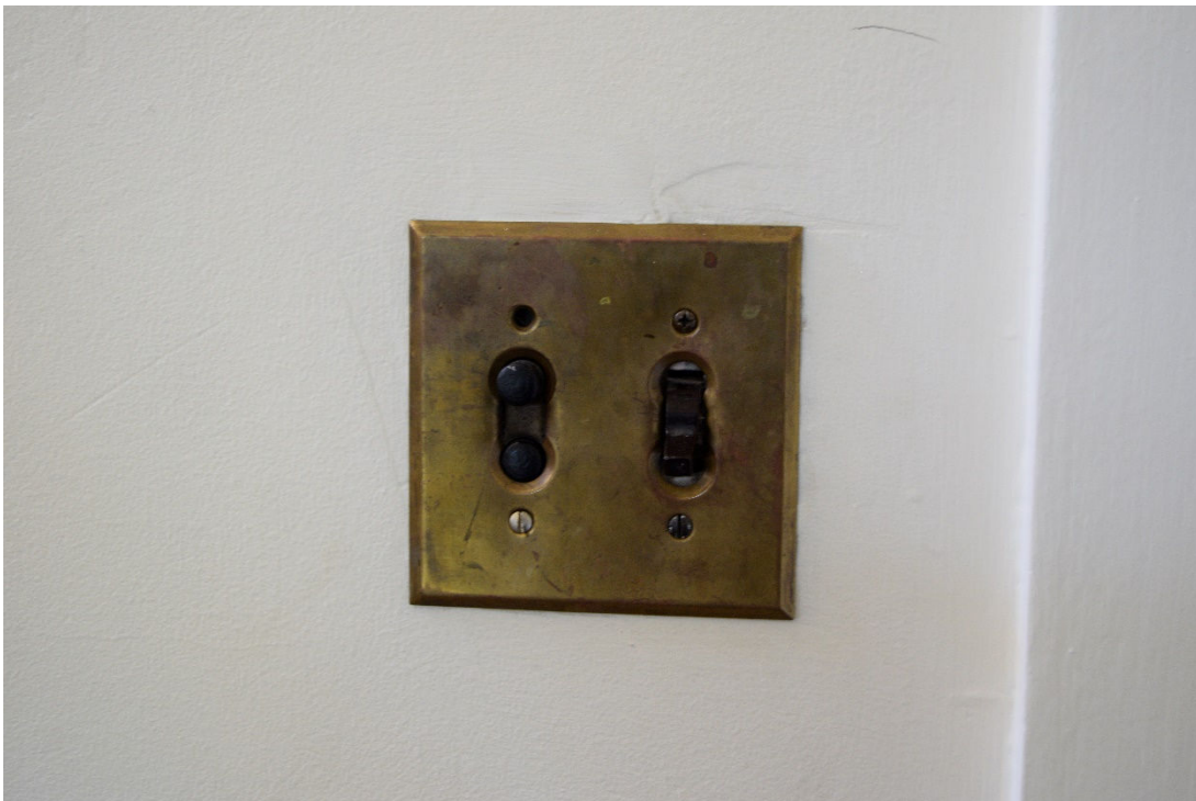
Image 38: Original push button light switch, knob and tube electrical
