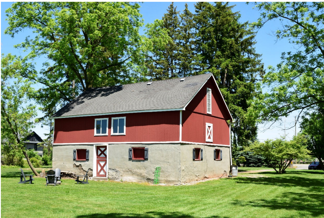
Image 41: West facade of outbuilding, note damage to parging, facing west
