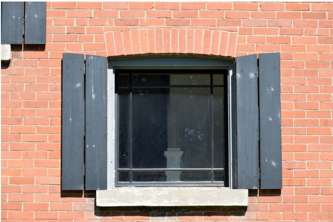
Image 6: Typical window with jack arch and cast lug sill, window and shutters are non-original
