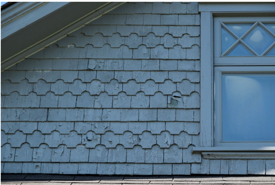
Image 7: Decorative cedar shakes used in gable ends, note condensation on windows indicating broken seals in need of replacement
