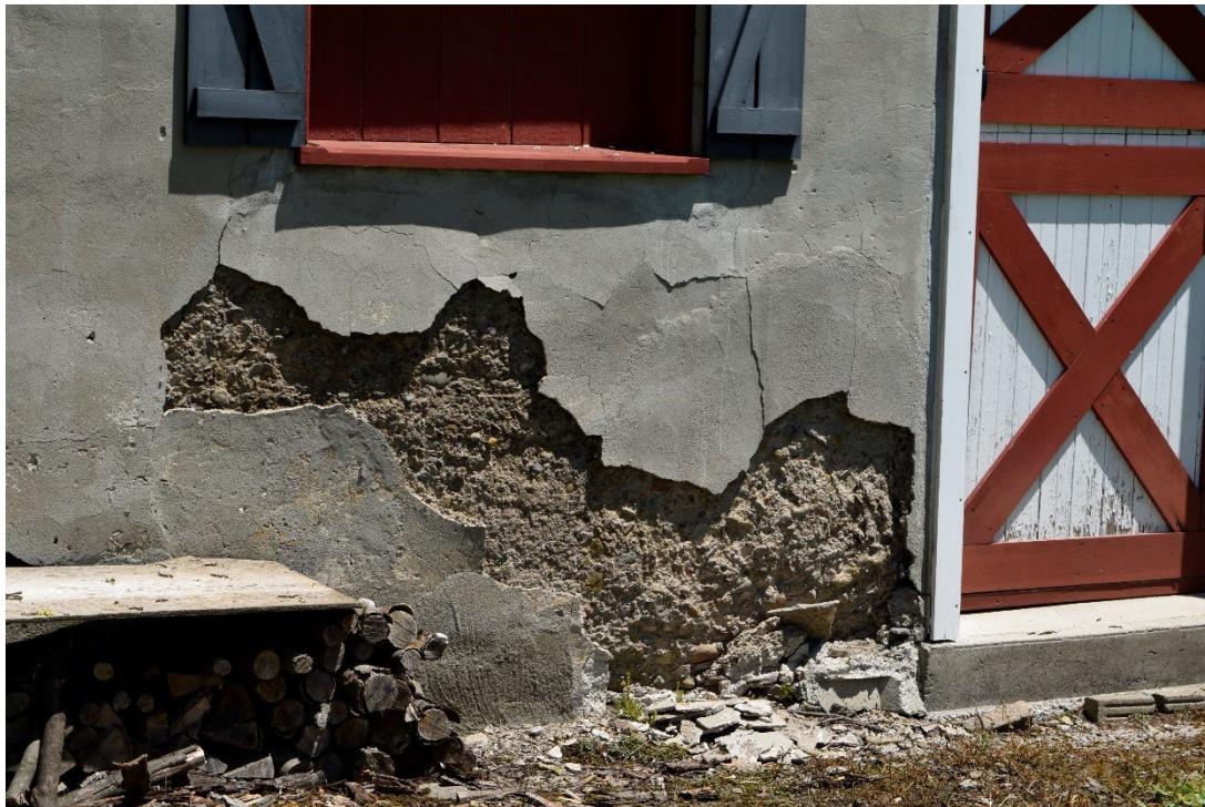
Image 43: Parge coat failing revealing coarse concrete foundation, note new concrete step associated with door
