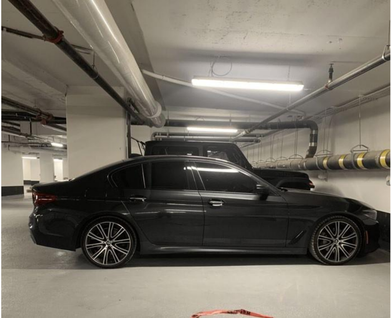
Parking Level A – Between V4 and V5 Jeep and sedan parked in space showing clearance to pipe with pipe height at its lowest of 1.24 metre from ground
