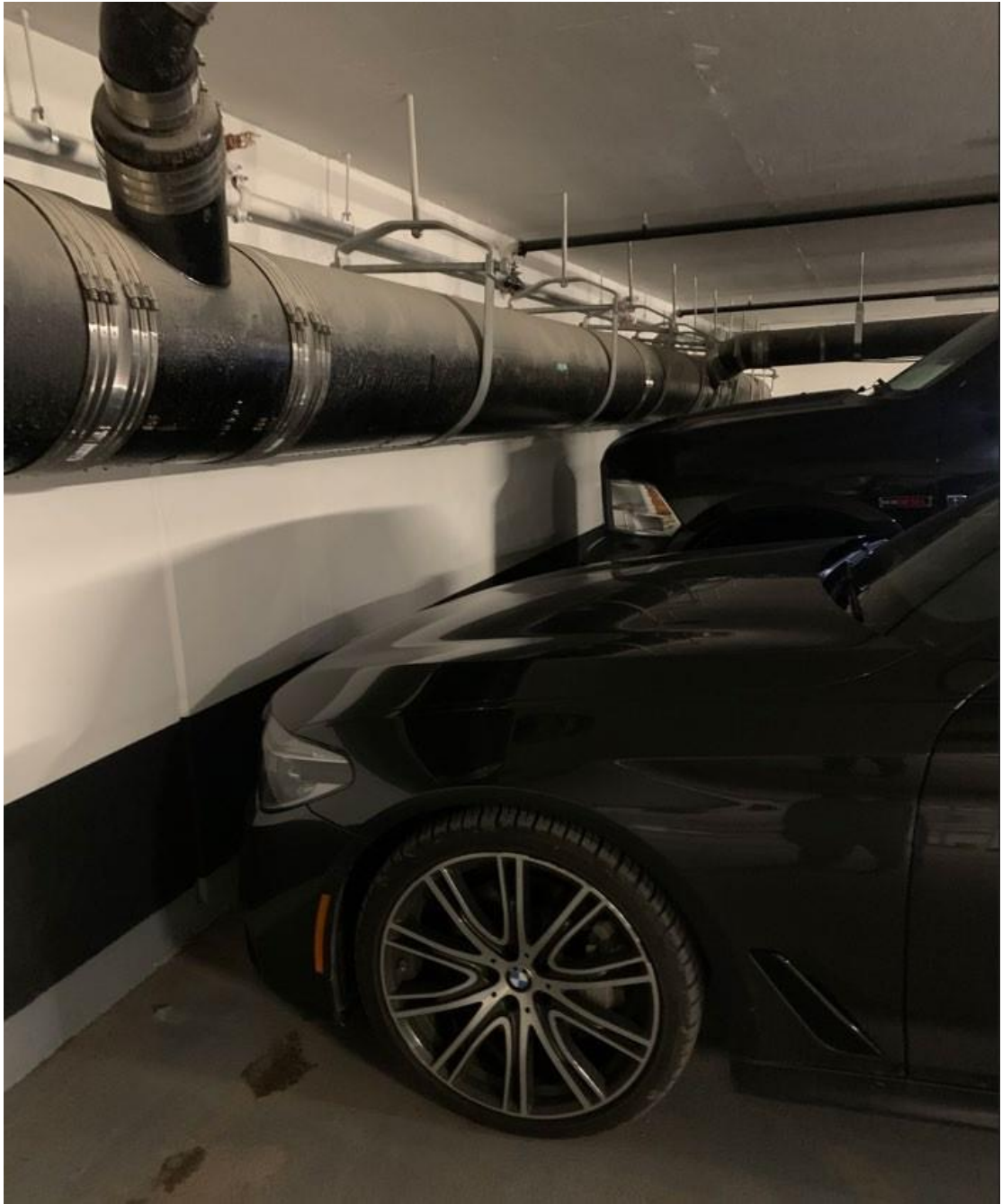
Parking Level A – Space 47 and 48 Vehicles parked in spaces clear of pipe including Ram 1500
