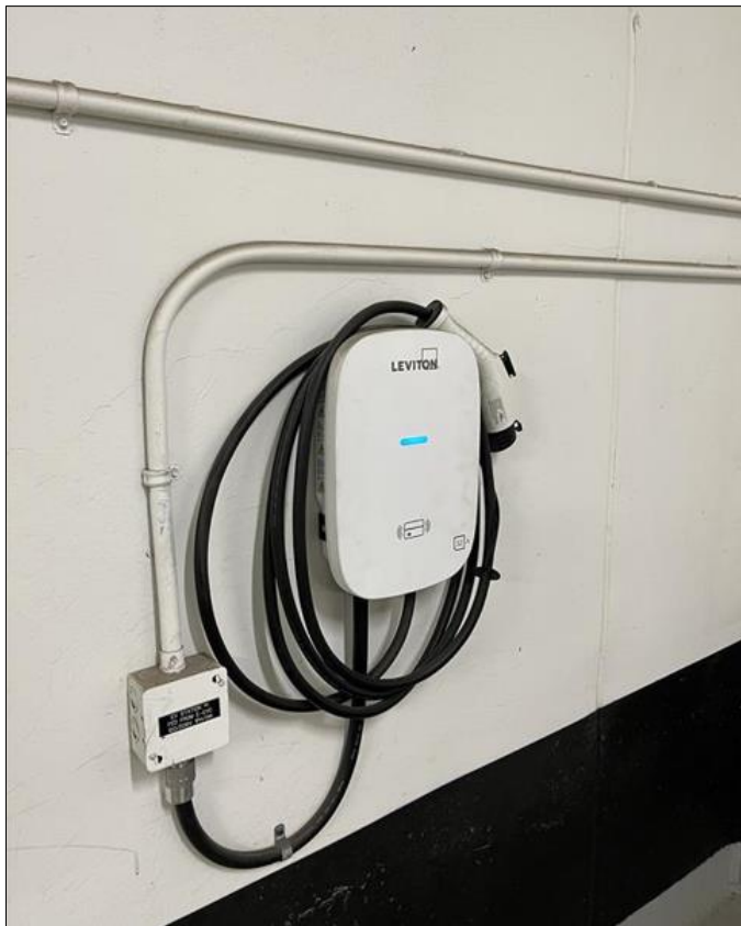
Figure 7 Installed Leviton Level 2 Wall Mounted Charger
