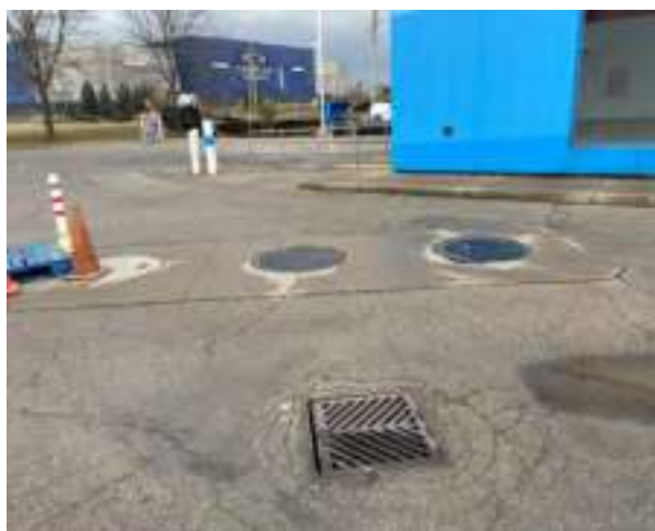
Photo 10 Comments: Interceptor beside the car wash station to the west.
