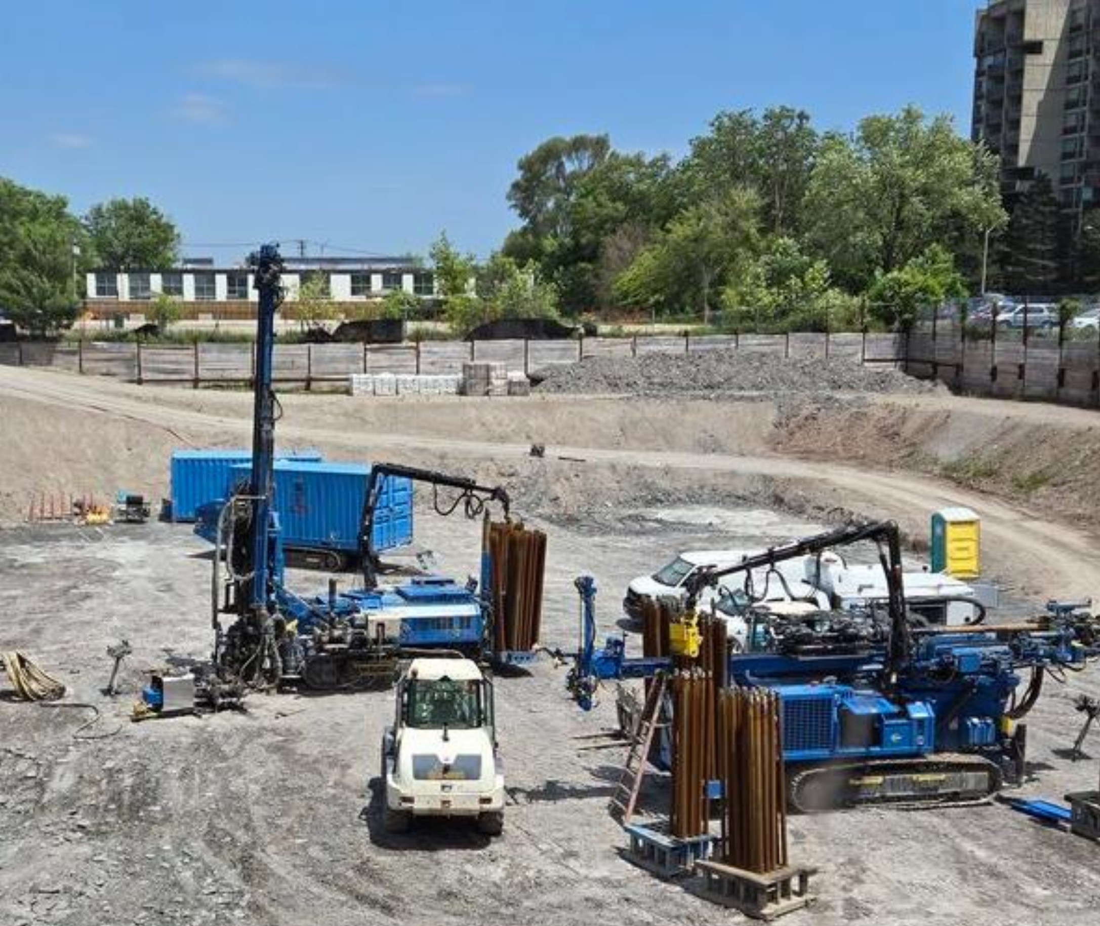
Pictured: The geo-exchange drilling at the new Gemini Condo development, part of the South-Oakville Kerr Village redevelopment plan
