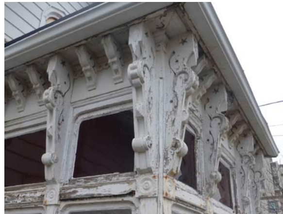
Showing deterioration of wooden decorative elements on front porch (ERA, 2017).
