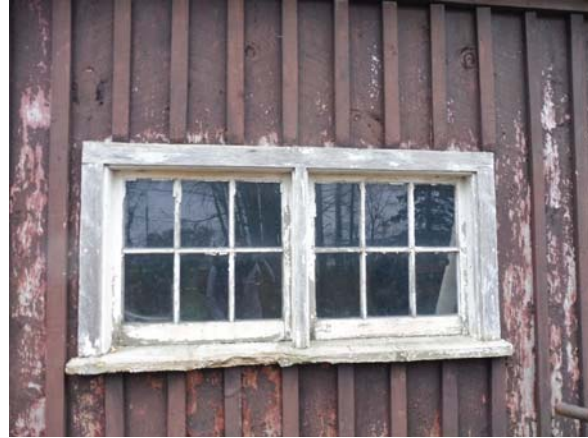
Showing wood deterioration, typical (ERA, 2017).
