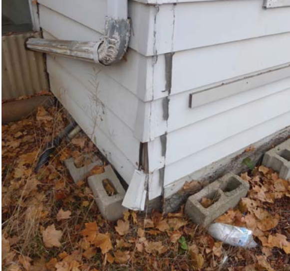
Showing wood rot to cladding substrate and sections of vinyl siding in poor condition (ERA, 2017).
