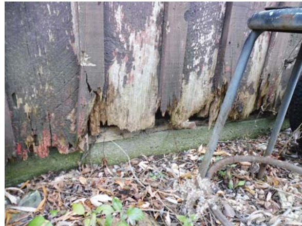
Showing wood rot of board and batten at grade (ERA, 2017).
