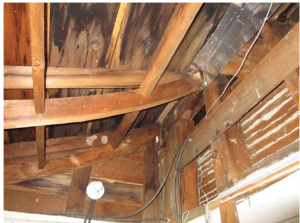
Bowed roof rafters(ERA, 2018).
