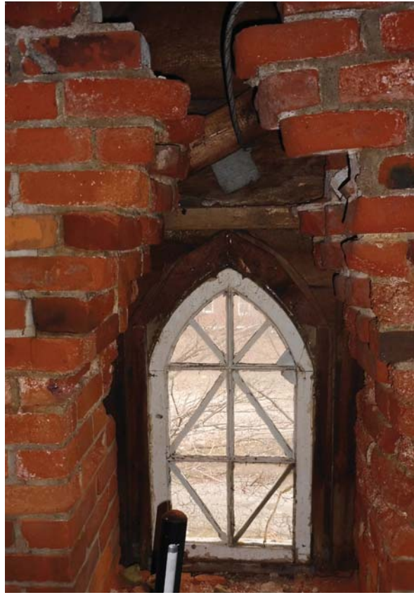
Showing original lancet window in attic in good repair, and brickwork in poor condition (ERA, 2017).
