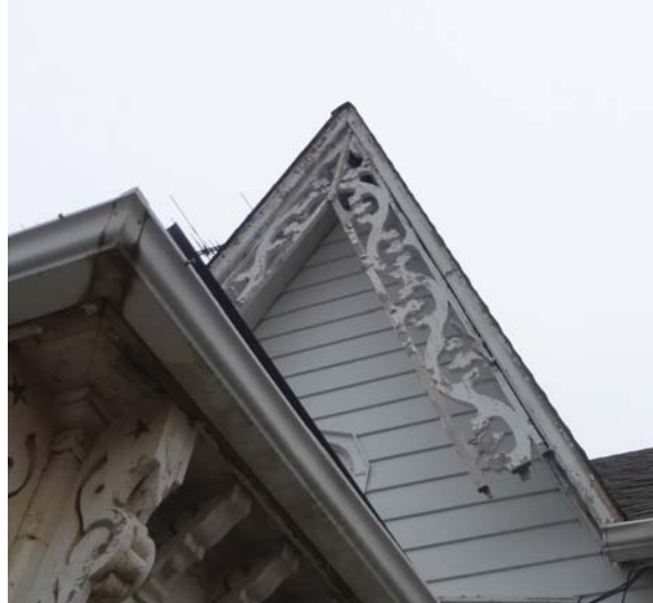
Showing wood rot and missing bargeboard (ERA, 2017).
