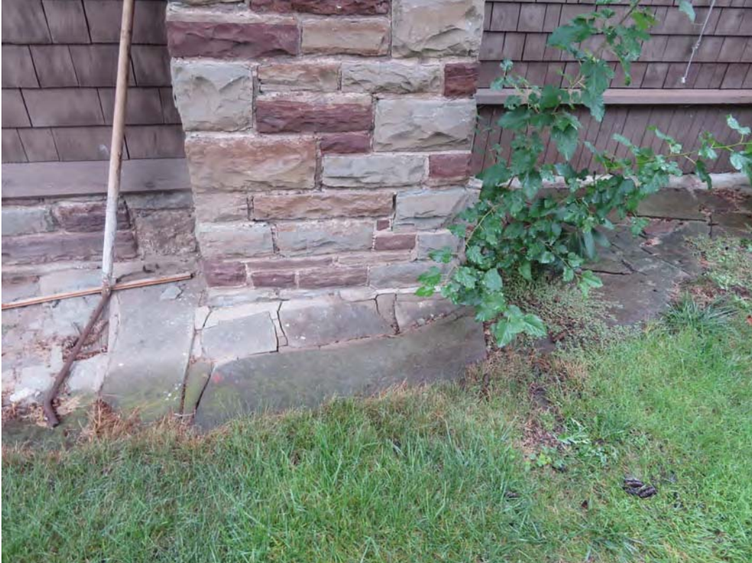
Flagstone paving – loose and missing mortar at the base of the masonry pier
