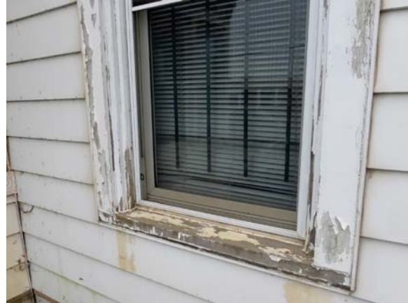
Paint flaking and deterioration of wood surrounds, typical (ERA, 2017).
