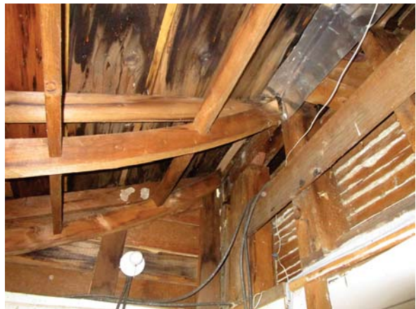
Bowed roof rafters(ERA, 2018).
