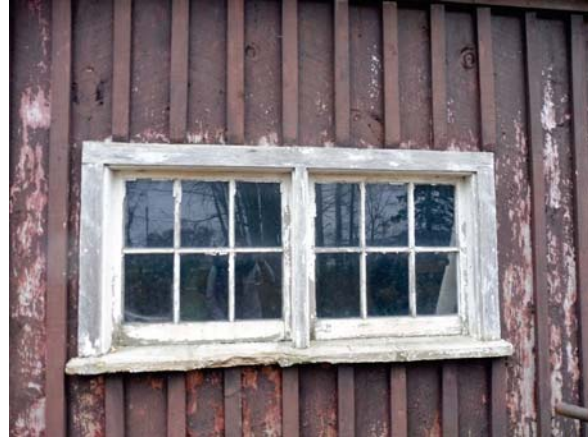
Showing wood deterioration, typical (ERA, 2017).
