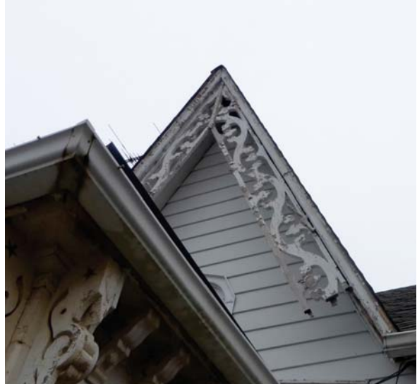
Showing wood rot and missing bargeboard (ERA, 2017).
