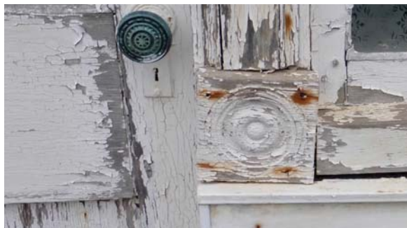
Porch details in poor condition (ERA, 2017).
