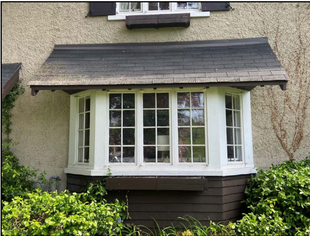
Exposed wooden eaves on the roof over the front bay window on the west elevation, 2024. This is the same on all overhanging rooflines of the house. Source: Town of Oakville Planning Staff
