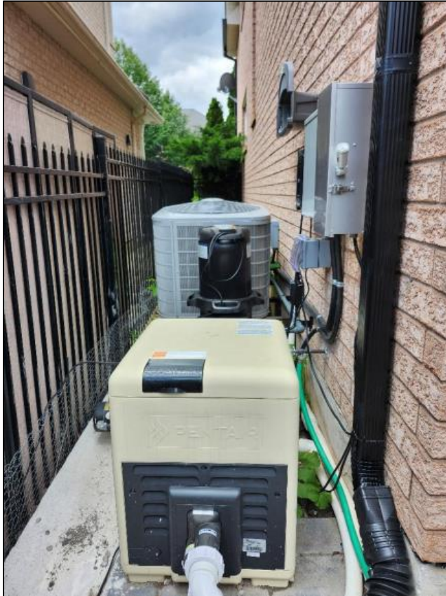
Existing Air Conditioner and Pool Equipment – 2255 Kingsmill Crescent
