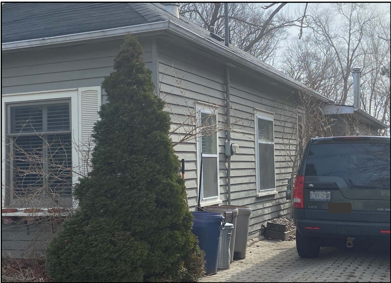
West elevation of the house, 2024. Source: Town of Oakville, Planning Services staff photo
