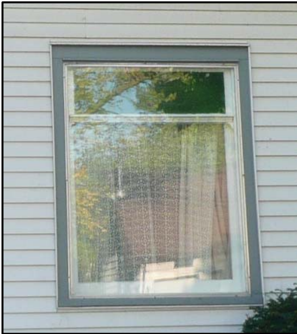
Close-up of one of the historic 1/1 wood sash windows, 2024. Source: Town of Oakville, Planning Services staff photo
