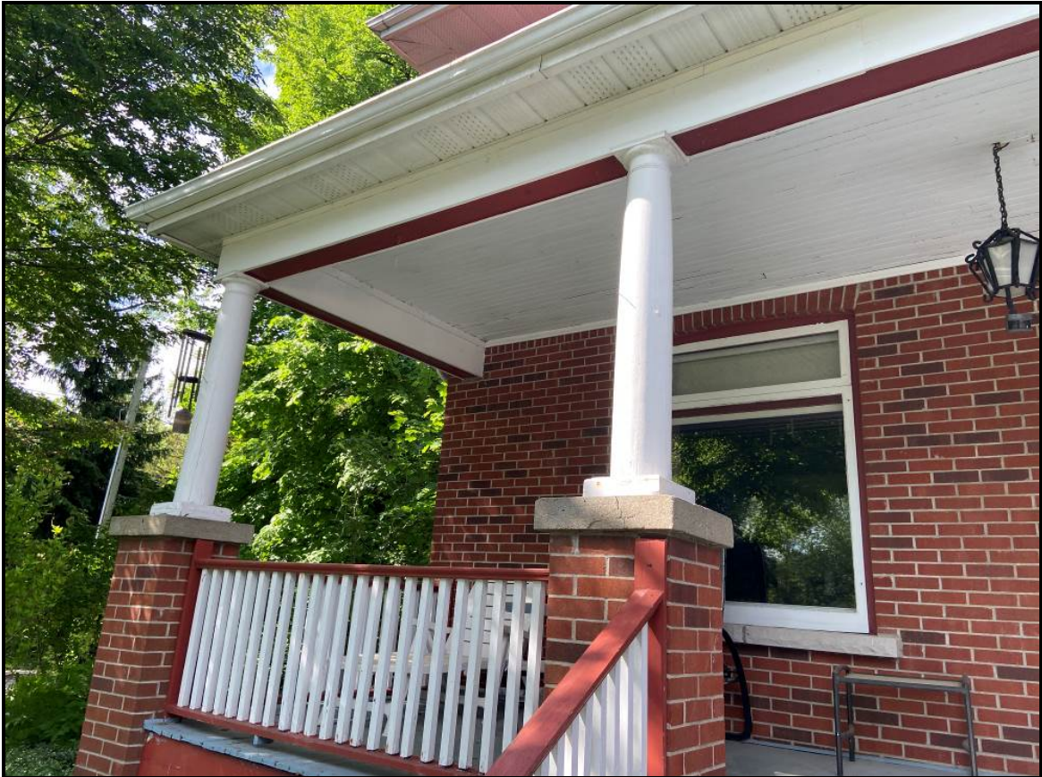
Close-up of two of the columns on brick piers, with the wooden ceiling and wooden architrave, 2024. Source: Town of Oakville Planning Staff
