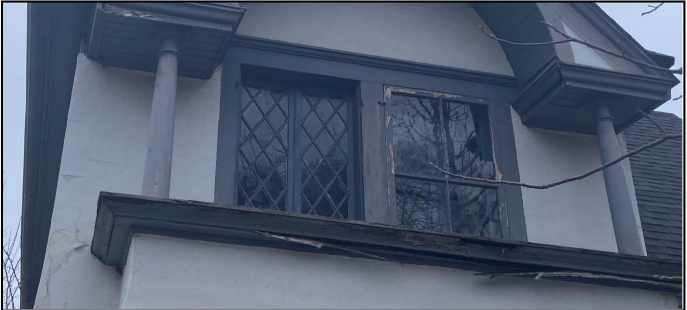
Upper-storey diamond-pattern windows. One is missing a storm window. Source: Town of Oakville Planning Services Staff
