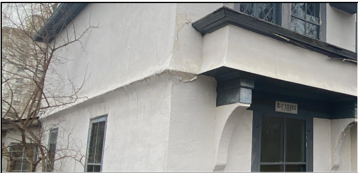
Close-up of the ledge. Source: Town of Oakville Planning Services Staff
