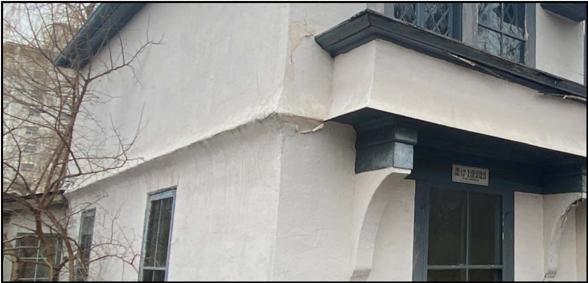
Close-up of the ledge. Source: Town of Oakville Planning Services Staff
