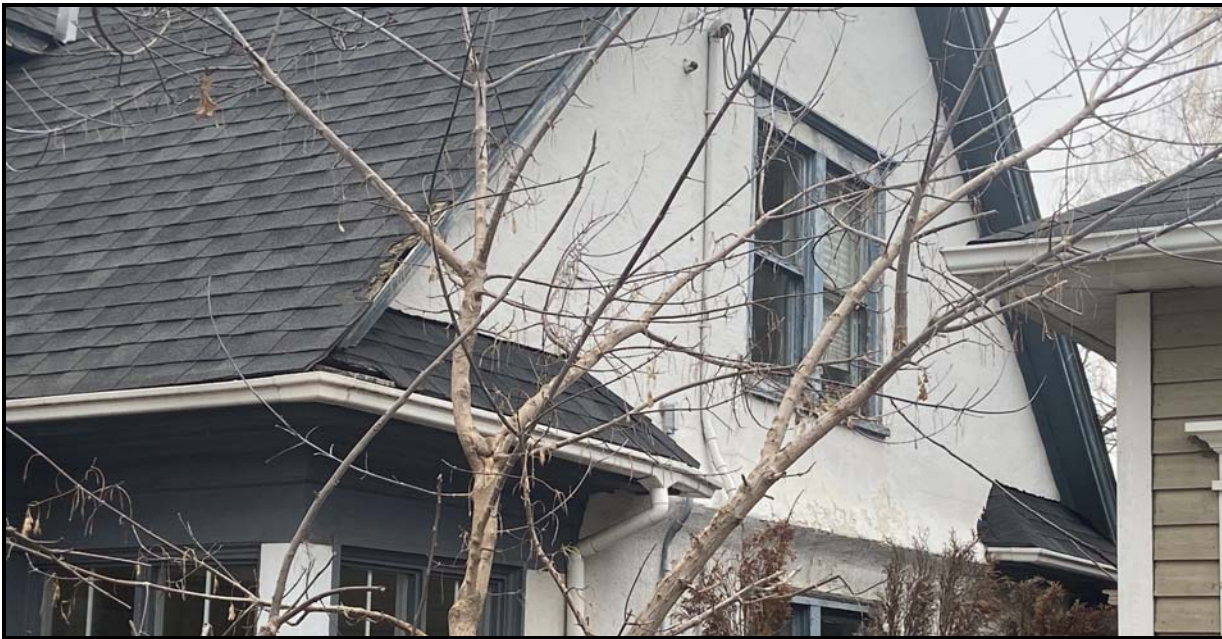
Side gable roof on the south elevation with roof-style returns, 2024. Source: Town of Oakville Planning Services Staff
