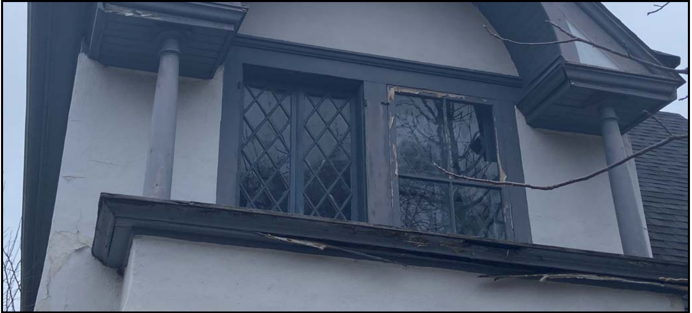
Upper-storey diamond-pattern windows. One is missing a storm window. Source: Town of Oakville Planning Services Staff
