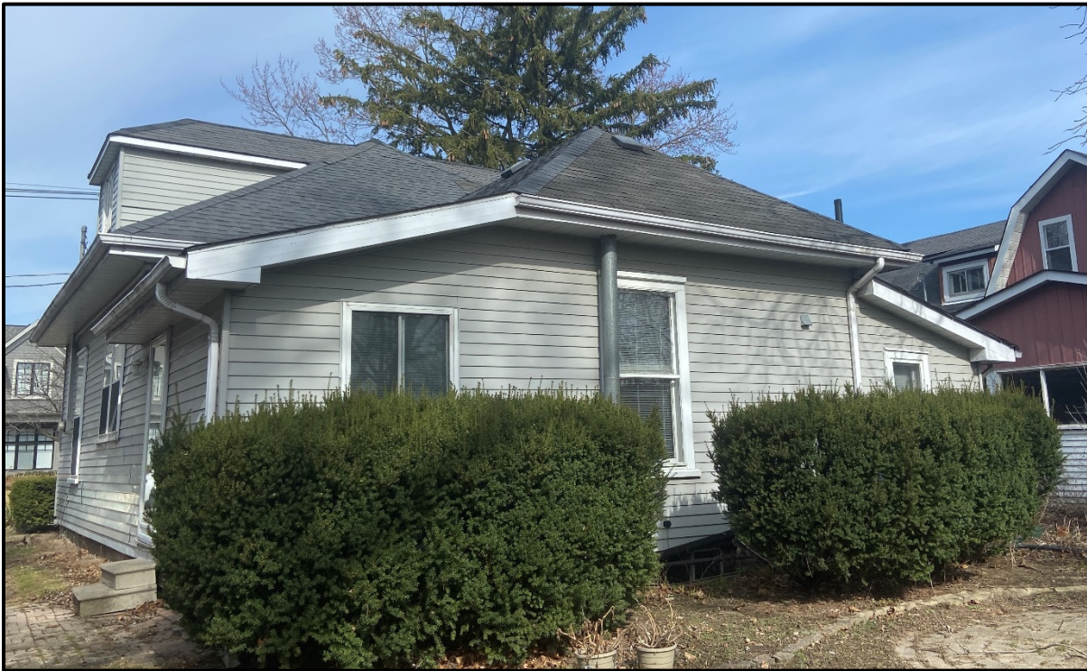
South elevation of the house showing rear wings added to the original house, 2024. Source: Town of Oakville, Planning Services staff photo
