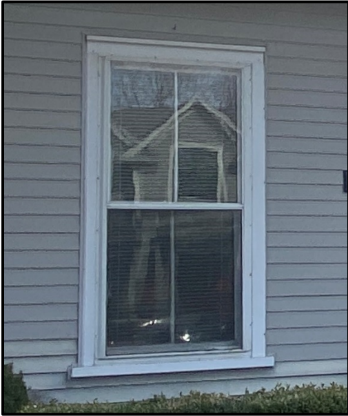
Close-up of one of the historic 2/2 wood sash windows, 2024. Source: Town of Oakville, Planning Services staff photo
