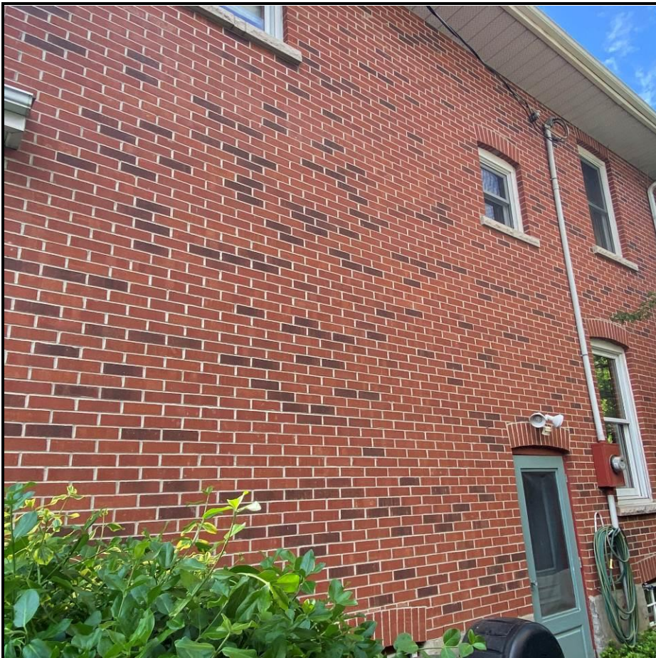
Close-up of the running bond brick pattern, 2024. Source: Town of Oakville Planning Staff
