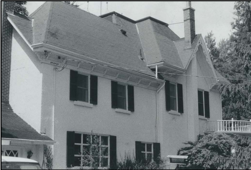
1977 photo showing the thick wooden muntins and square panes of glass on the first storey windows. Source: Town of Oakville planning files
