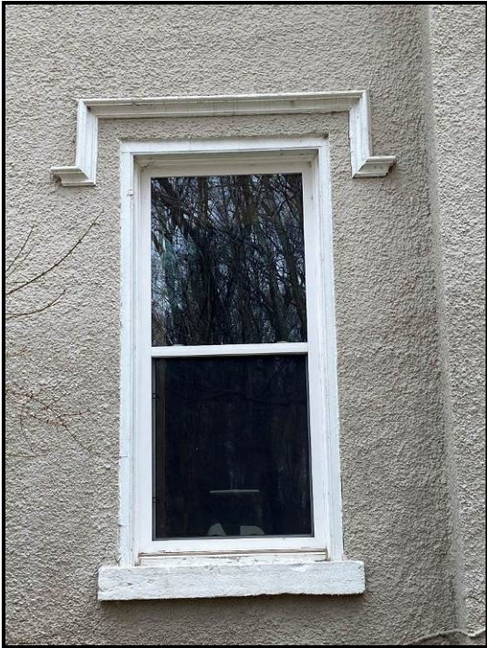
Close up of one of the windows with drip edge on the north elevation, 2024. Note the wood sills and frame. Source: Town of Oakville Planning Staff
