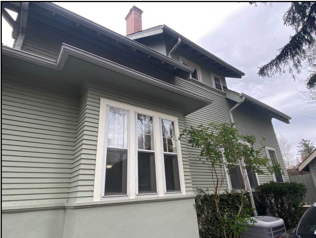
West elevation fenestration with projecting window, 2024. Source: Town of Oakville Planning Staff
