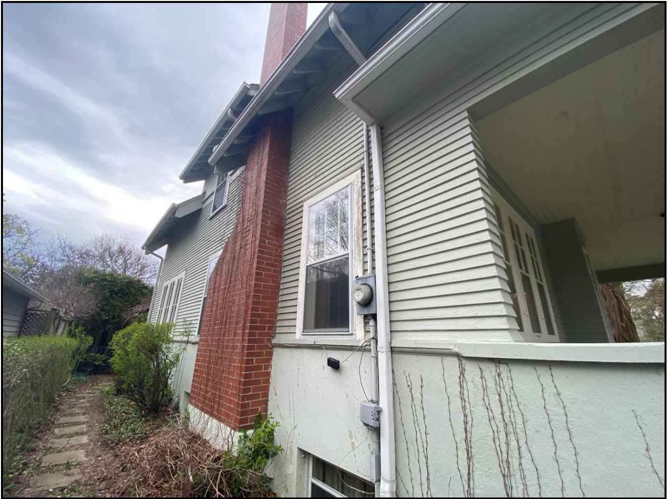
East elevation showing the shed dormer, chimney, porch overhang, and fenestration, 2024. Source: Town of Oakville Planning Staff
