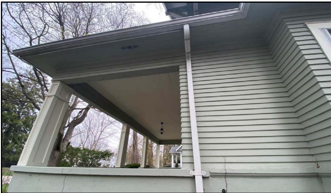
View of the front porch roof overhang with wooden soffit that goes around both sides of the house and acts as the roof on the projecting window on the west elevation, 2024. Source: Town of Oakville Planning Staff
