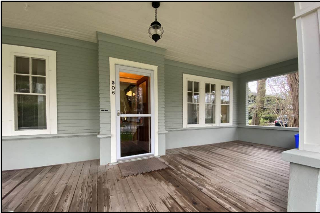
Front porch showing the wooden ceiling, flooring, the trim running along the foundation, and the projecting front door, 2024. Source: Town of Oakville Planning Staff
