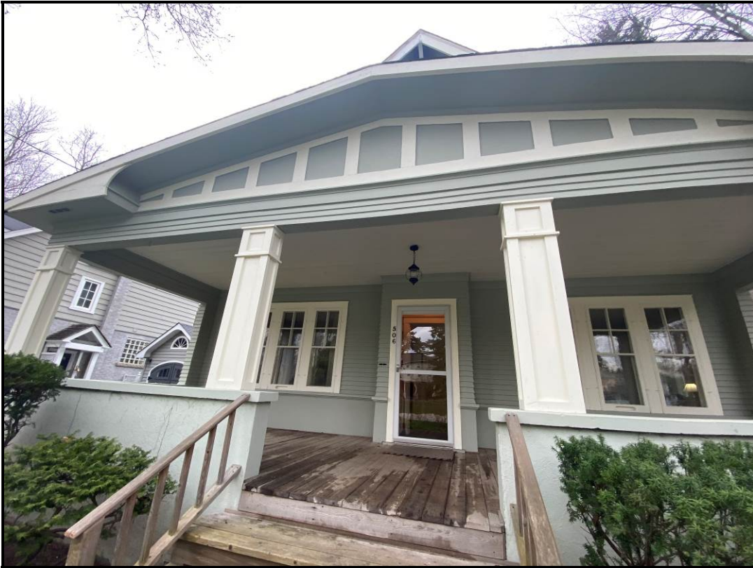
Wooden detailing on the porch showing the columns, half-timbering, the decorated edges, wooden trim detailing, and a concrete porch wall, 2024. Source: Town of Oakville Planning Staff
