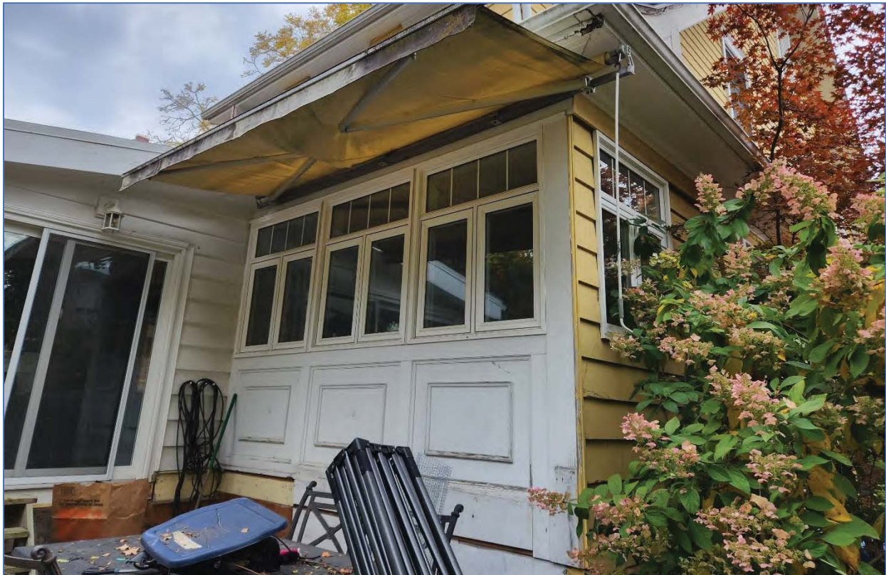
Photo 17: View northwest showing part of the northeast and southeast elevation of the first addition
