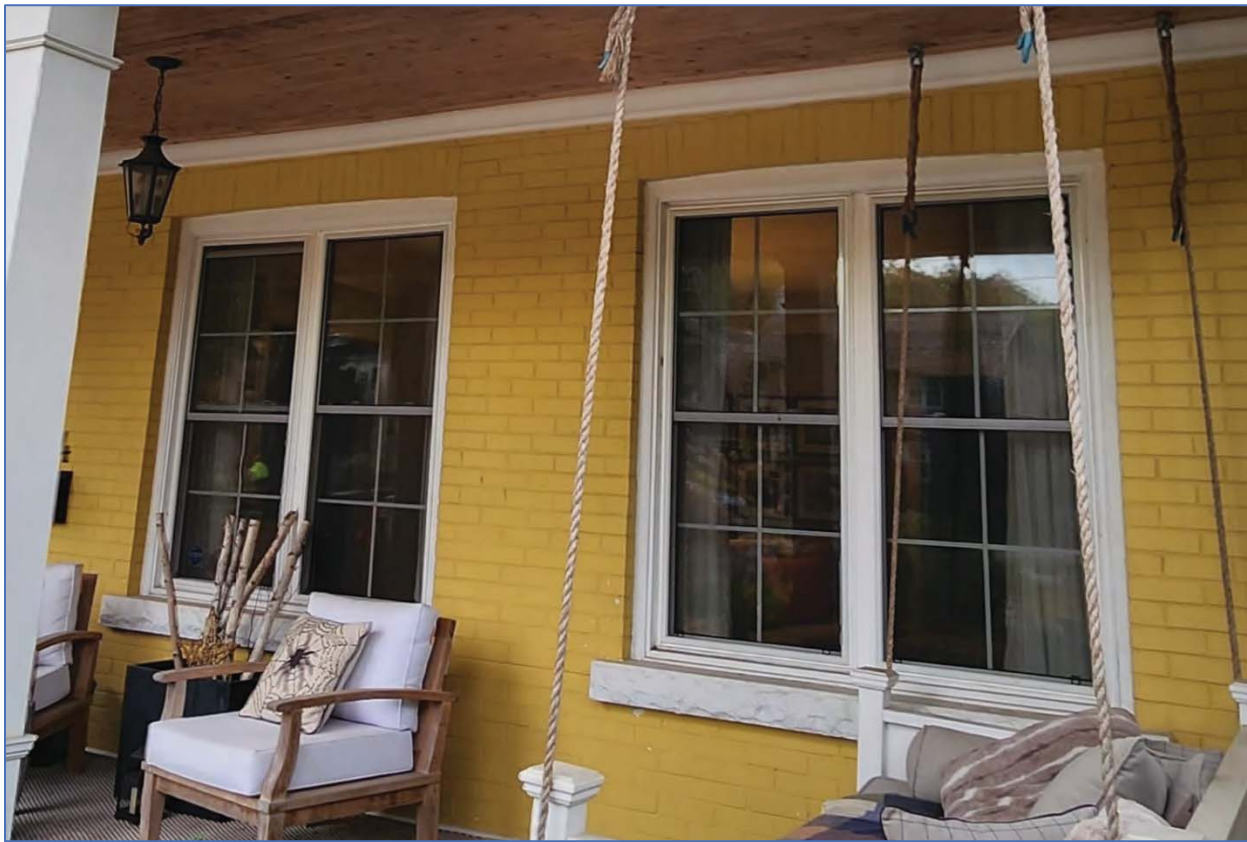
Photo 15: View east showing two typical first storey windows on the northwest elevation
