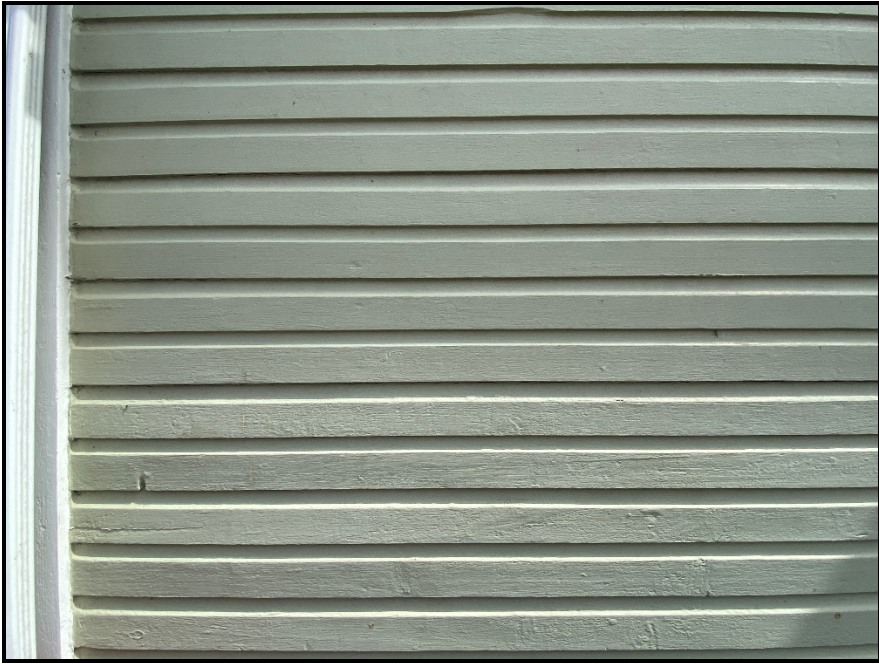
Close up of the wood horizontal siding, 2024. Source: Town of Oakville Planning Staff
