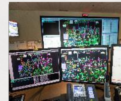
Control room services
