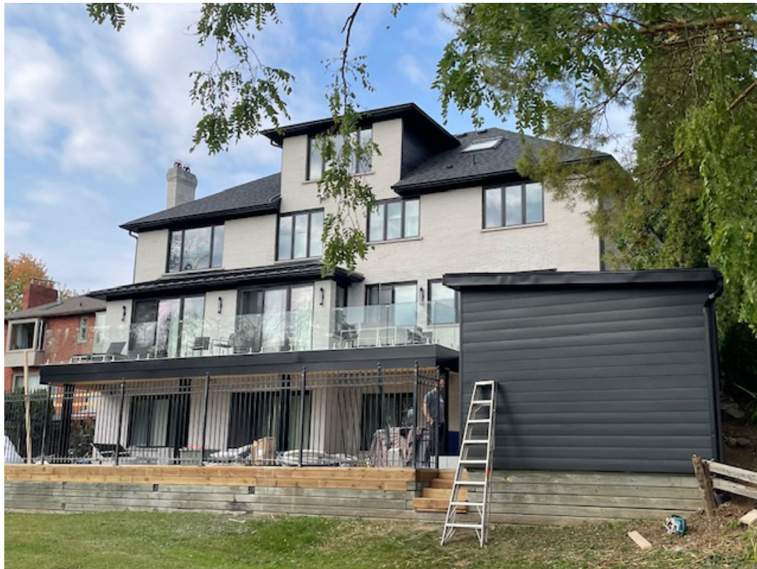
Photo of the rear yard after cosmetic renovations. The roof, windows, deck railing, paint and siding have been updated. Additionally, repairs have been made to the existing retaining wall and steps.
