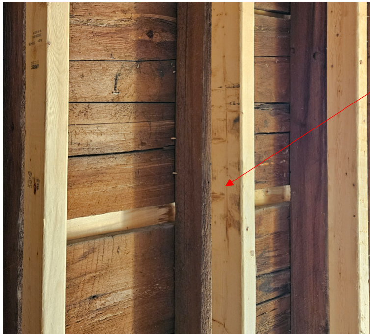
New stud wall at rear addition that is not fastened to the existing studs.
