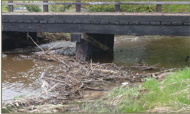
Debris in Creeks
