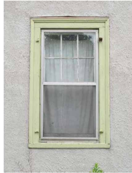
Ground floor window on north (principal) elevation of 42 Lakeshore Road West (ERA, 2011)
