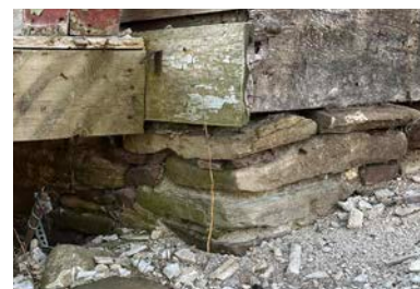
Deep mortar loss and loose stone along the foundation (ERA, 2023).
