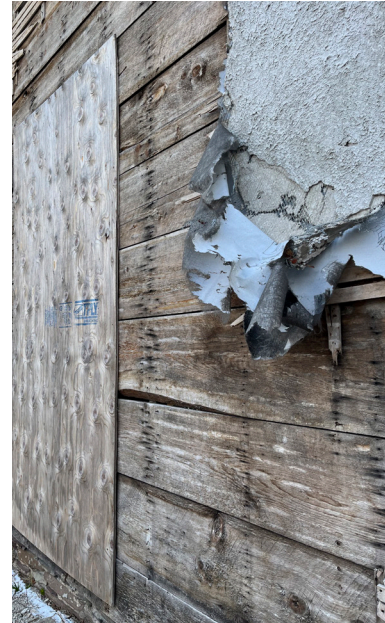
North elevation stucco, which is only partially remaining (ERA, 2023).
