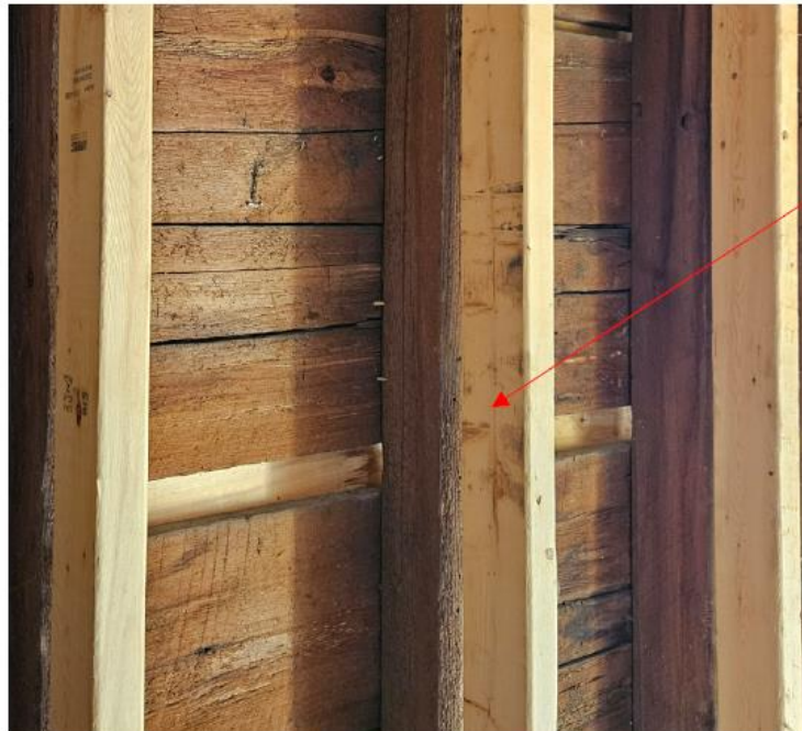
New stud wall at rear addition that is not fastened to the existing studs.
