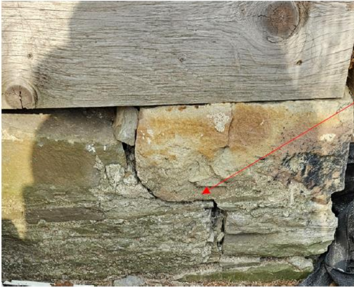
Crack on the south-east corner of the rubble foundation wall.
