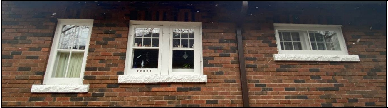
Wood windows on the north elevation. Source: Town of Oakville Planning Services Staff
