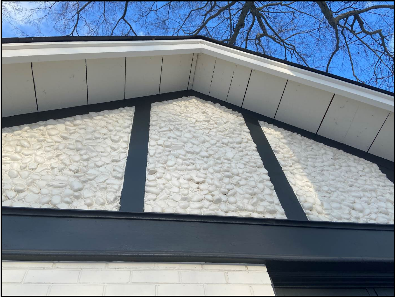
Pebbledash cladding on the front gable with half-timbering. It has been painted. Source: Town of Oakville Planning Services Staff
