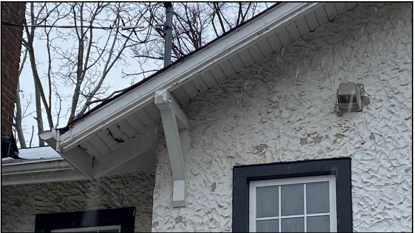
Close up of one of the wooden brackets that are spaced underneath the eaves, as well as wooden soffit and fascia. Source: Town of Oakville Planning Services Staff
