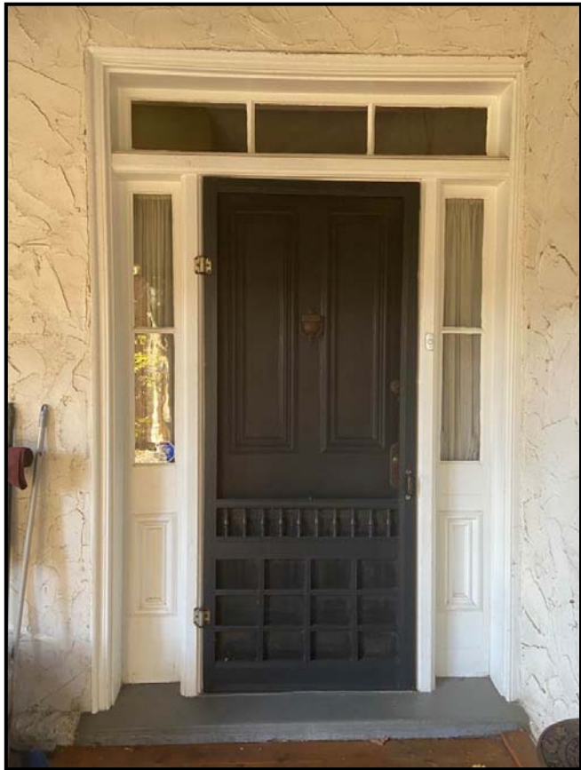
Front door showing the windows, the two-panel wooden door, and Victorian-style screen door. Source: Town of Oakville Planning Services Staff
