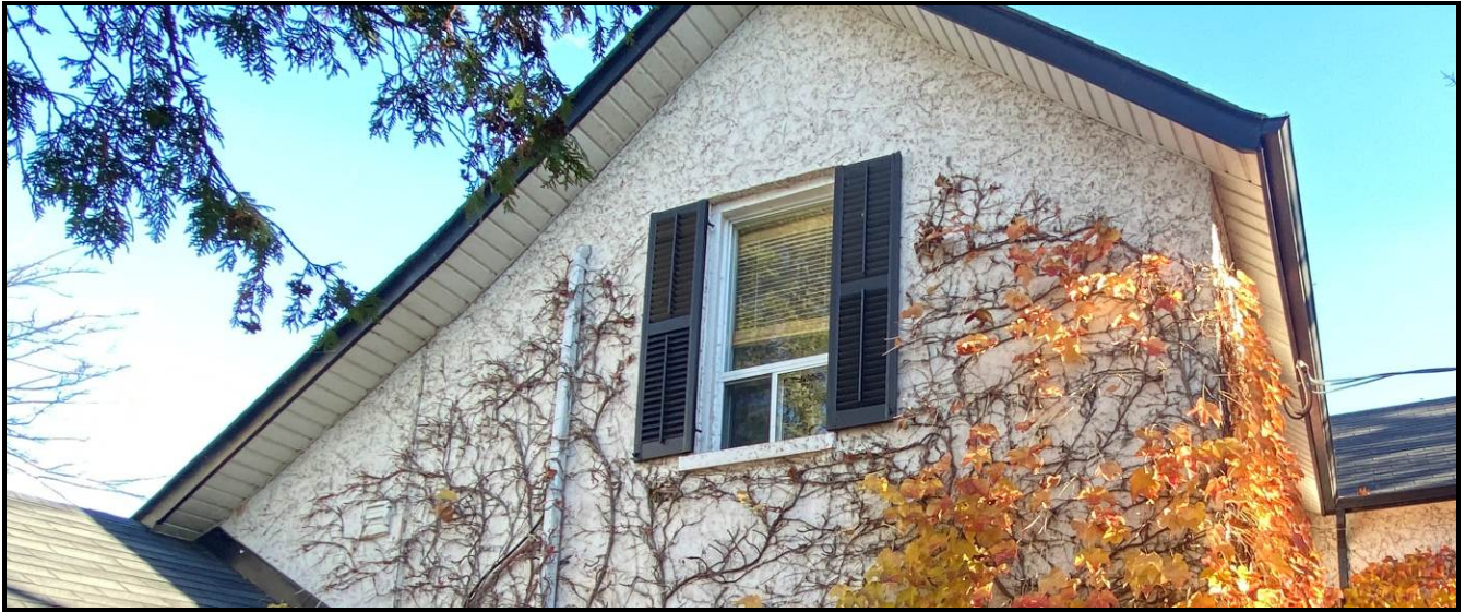
North elevation stucco, showing a pebbled appearance. It is similar to the stucco on the one-storey portion. Source: Town of Oakville Planning Services Staff
