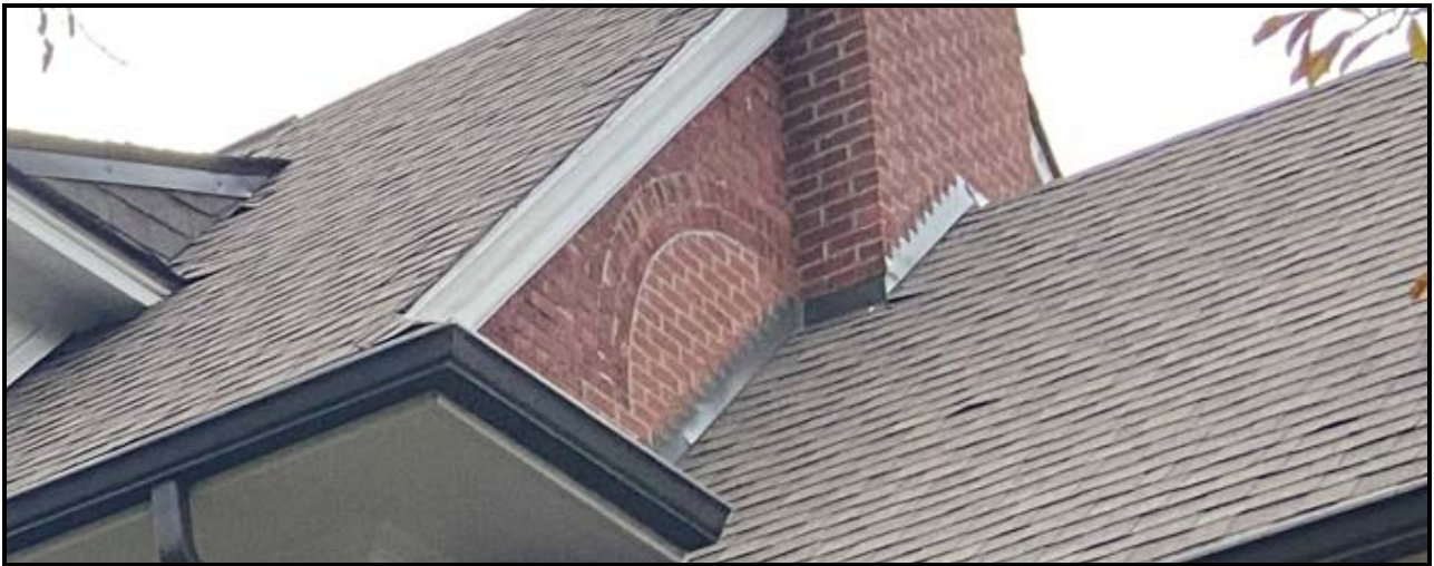
Bricked in quarter lunette windows on east elevation, indicating a once similar elevation to the west, with the bumpout most likely being only one storey. Source: Town of Oakville Planning Services Staff
