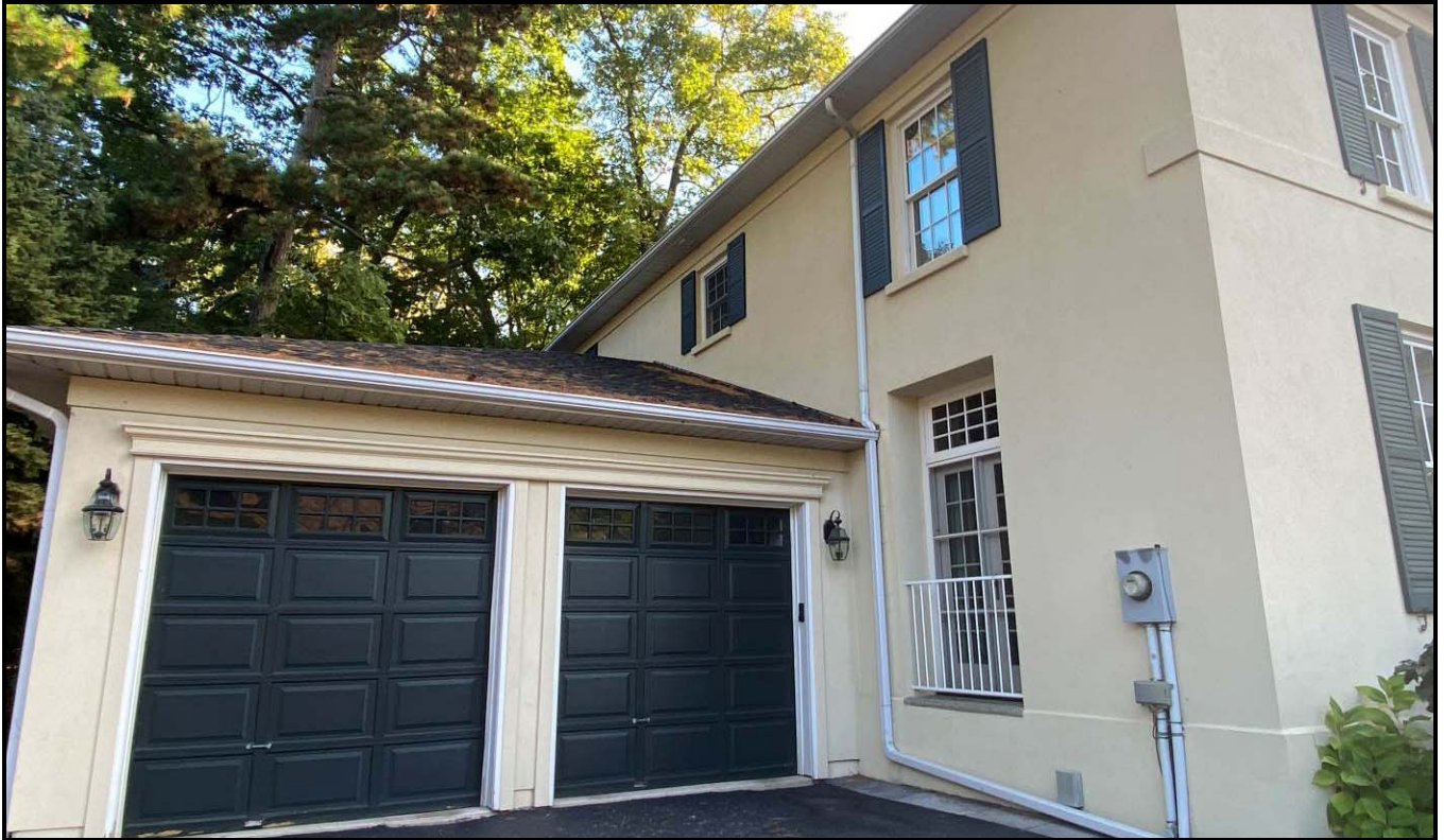
New garage built where the old south-facing two level porch addition had been built during the Stuart's ownership, and north elevation. Source: Town of Oakville Planning Services staff
