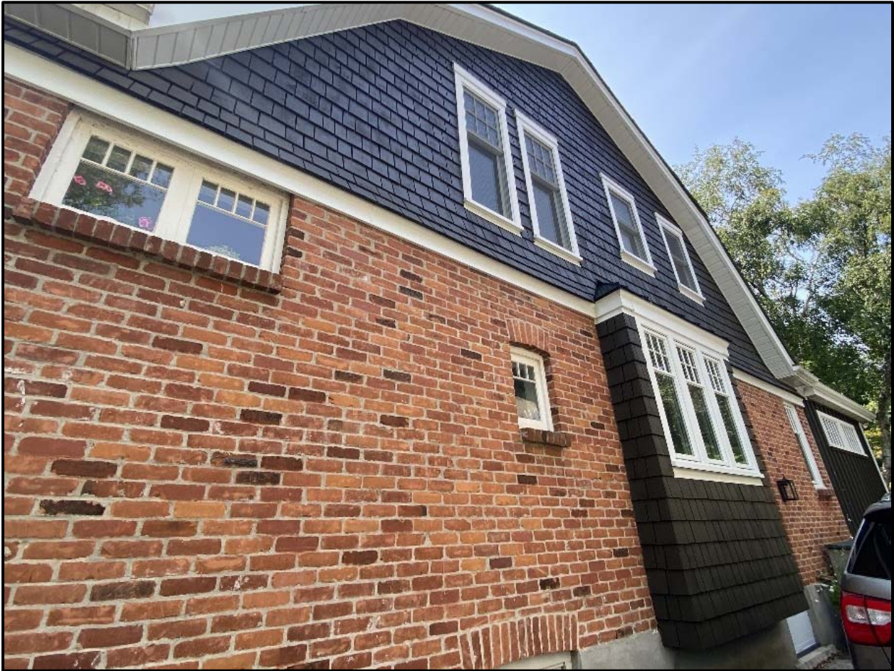
East elevation, showing some of the variety of windows used on the Cuthbertson House. Source: Town of Oakville, Heritage Planning staff photo
