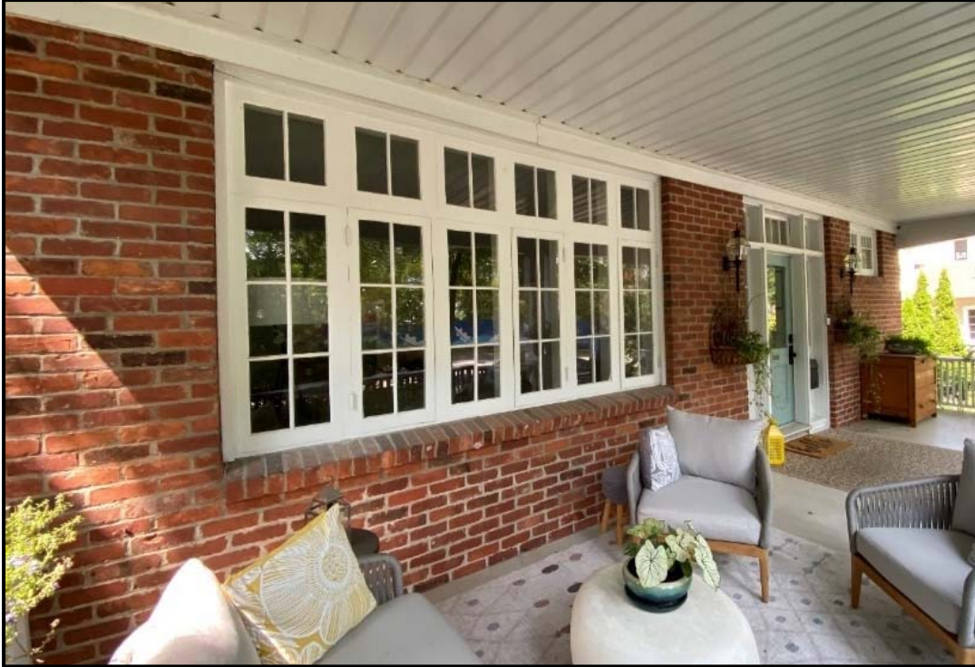
The south, or front, façade, includes early paired casement windows with functional wood muntin bars. Source: Town of Oakville, Heritage Planning staff photo
