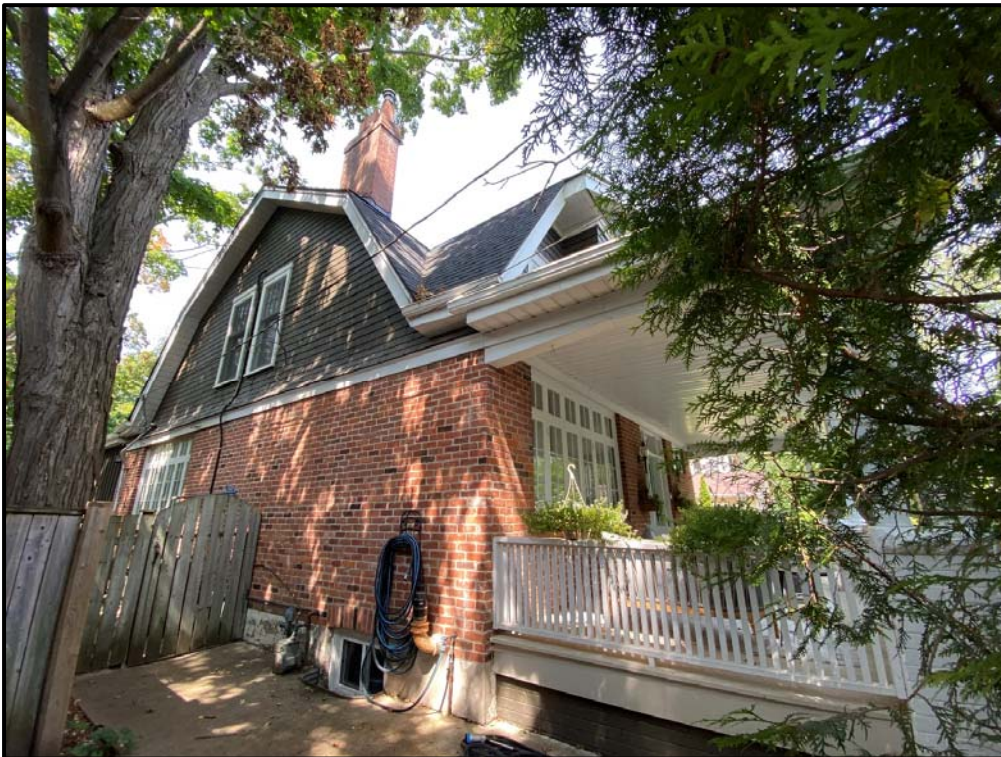
The west elevation includes the house's only chimney. Source: Town of Oakville, Heritage Planning staff photo
