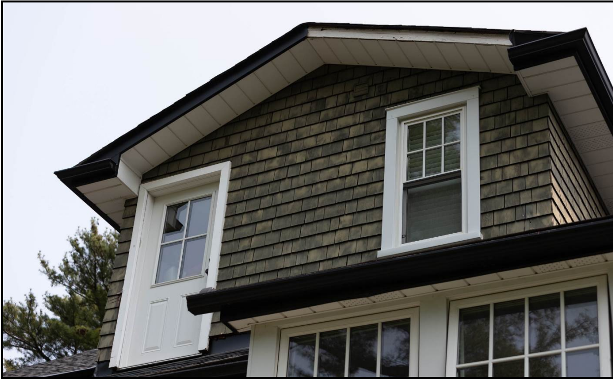
The door on the rear dormer would have been added later when the third-storey apartment was constructed for the external stairs evident in the 1998 survey. Source: Town of Oakville Planning Services Staff
