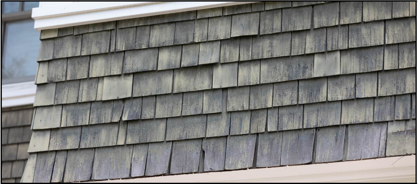
Close up of the wooden shingles on the west elevation of the house. Source: Town of Oakville Planning Services Staff
