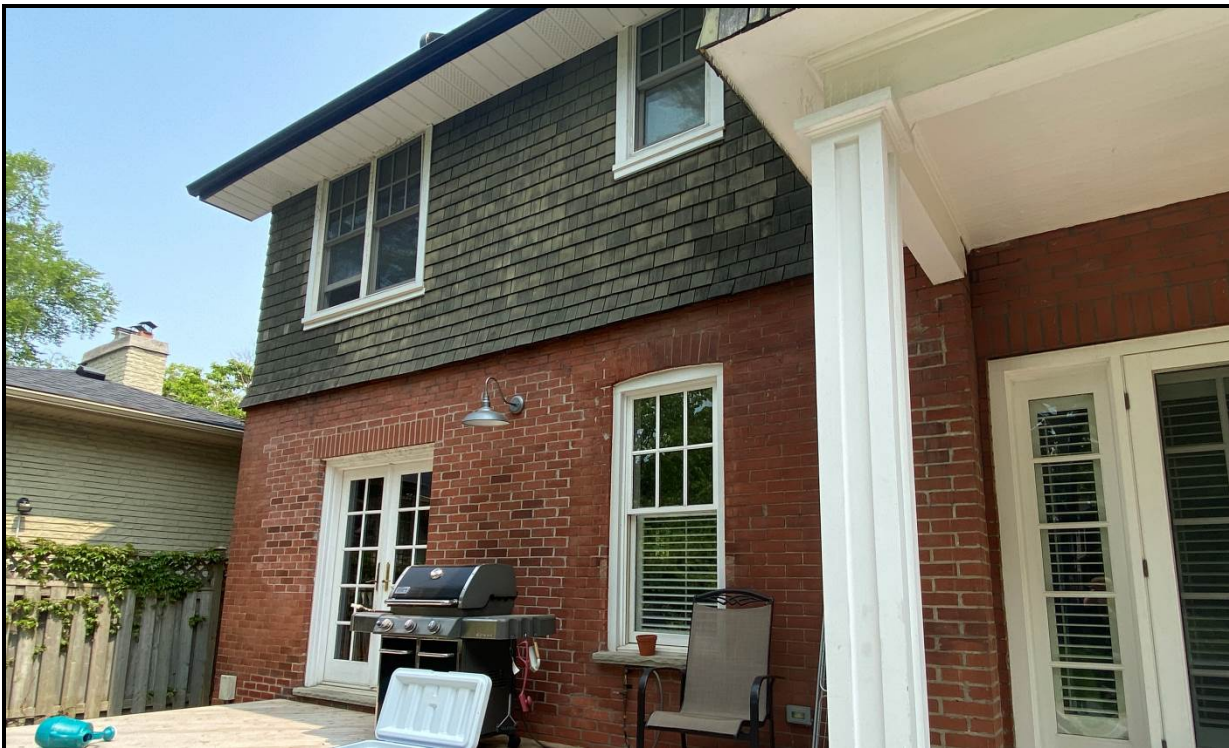
6/1 windows on the west (rear) elevation of the home. The French doors were added later as evident by the updated brick work. It is unknown what was there previously. Source: Town of Oakville Planning Services Staff
