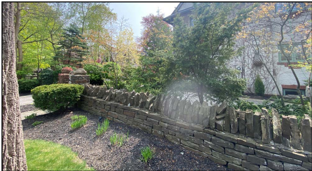
Photos of the lakestone wall in front of 330 Watson Avenue. The column cap stones are slightly different than those on Douglas Avenue and it appears they have been worked on at some point and some stones have been mortared. The owners of the home have also found old iron gate hardware. Source: Town of Oakville Planning Services Staff
