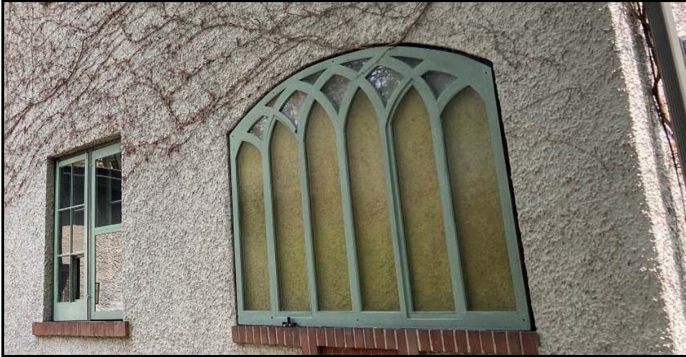
North elevation of the home with garage to the left. We can see the covered window on the right that would have originally been an opening of the covered porch. Source: Town of Oakville Planning Services Staff
