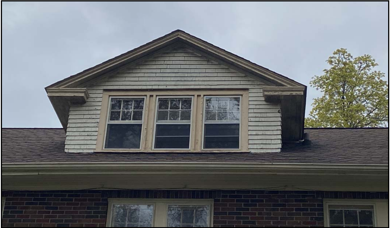
Close up of dormer on southern elevation (façade), with wooden shingles and wooden soffits.
