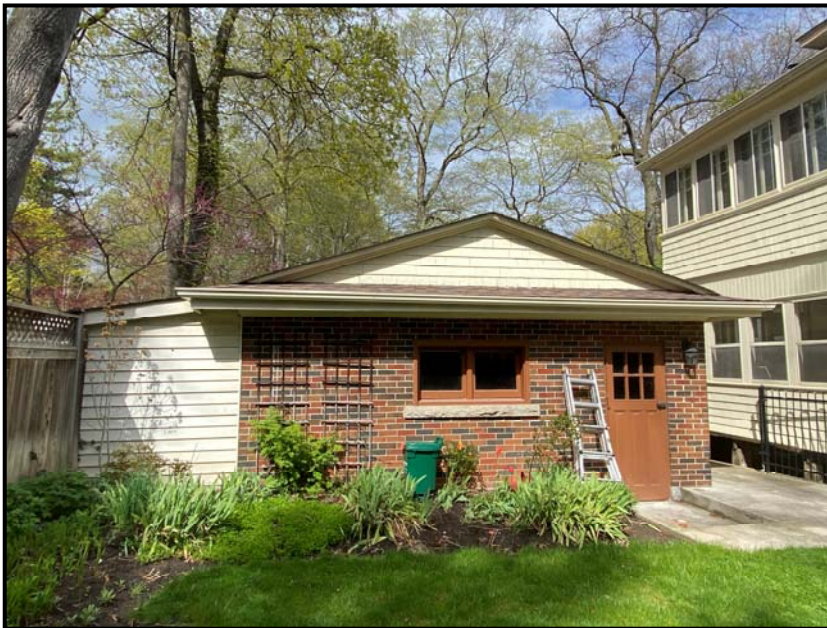
Rear of the garage, looking east. A greenhouse was once attached on this side.
