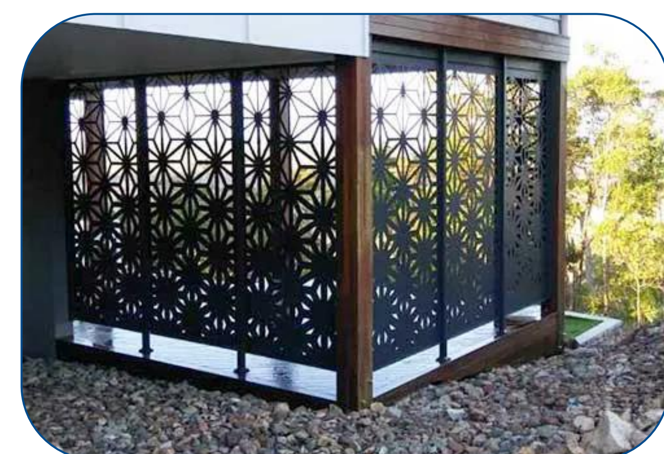
Utility policies direct that new services are provided underground, interior to the site and/or screened from the public realm. (Policy 20.5.1 (d))
