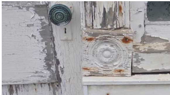
Porch details in poor condition (ERA, 2017).
