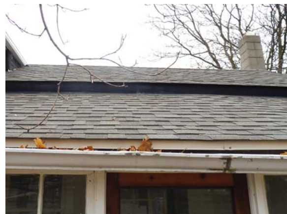
Asphalt shingles in good repair; gutters and downspouts requiring maintenance (ERA, 2017).
