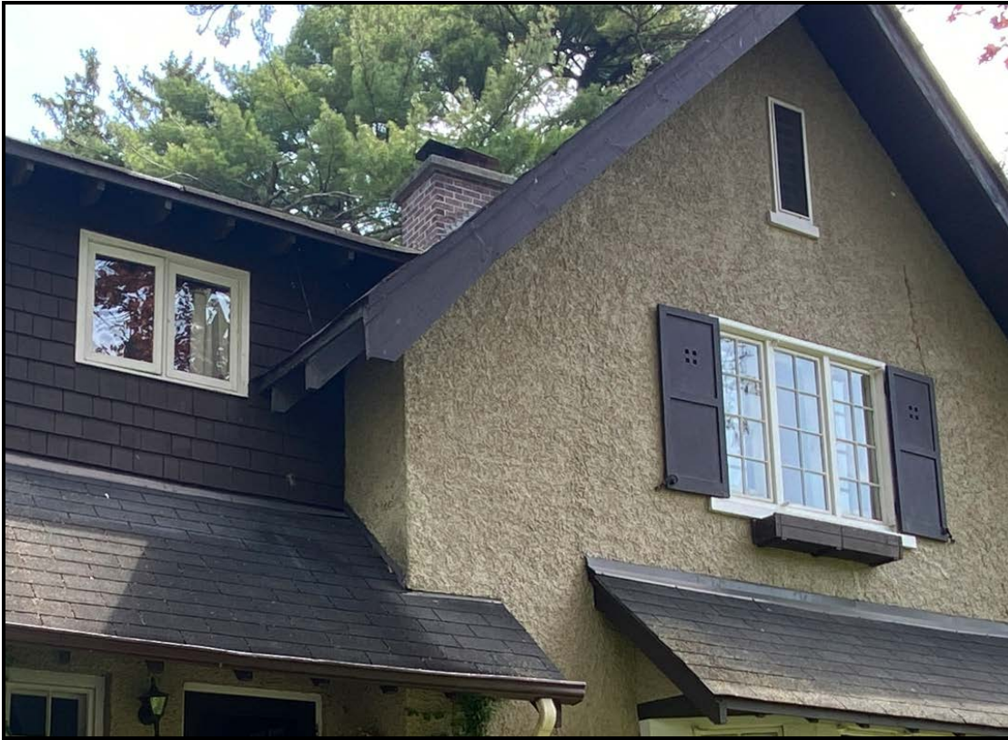
Close-up of the wooden fascia, soffit, and exposed eaves on the west elevation, 2024. Source: Town of Oakville Planning Services Staff
