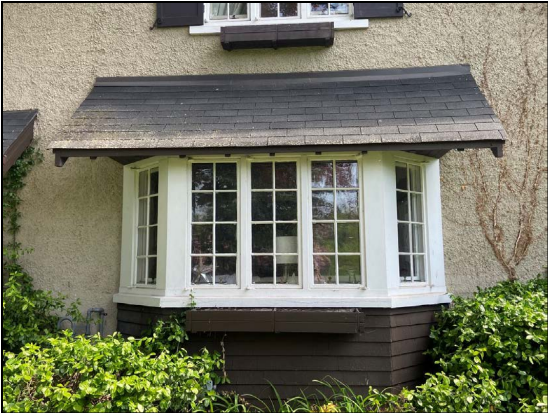
Exposed wooden eaves on the roof over the front bay window on the west elevation, 2024. This is the same on all overhanging rooflines of the house. Source: Town of Oakville Planning Staff
