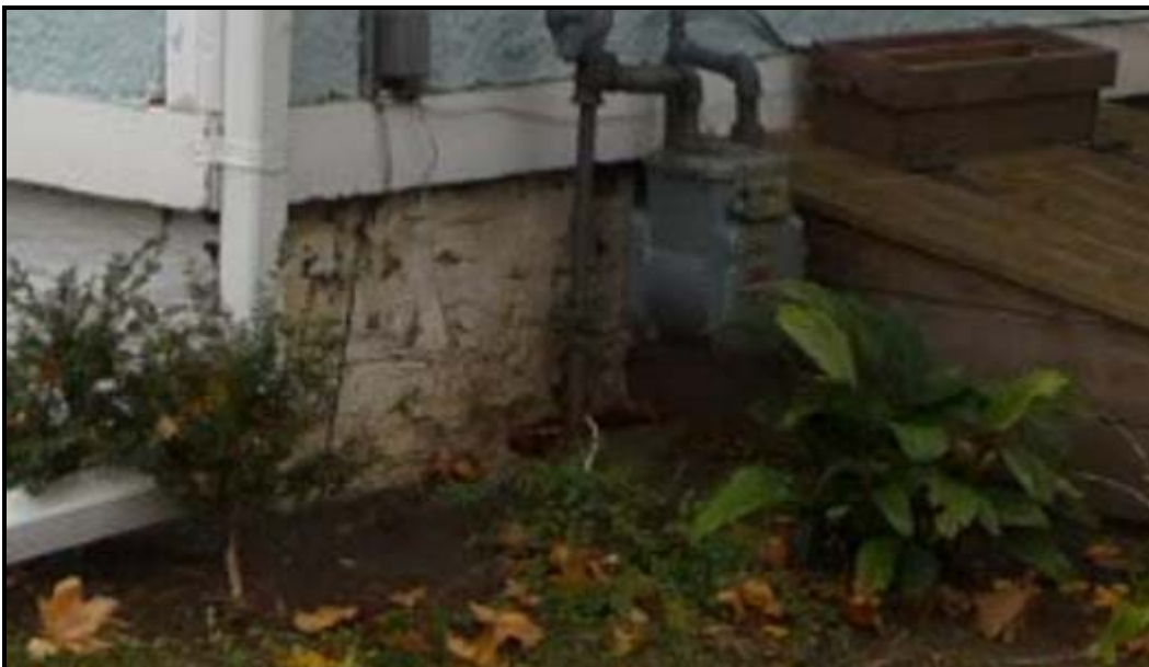
Close-up of the lakestone foundation, partially parged over. Source: Planning Services staff photo, 2008.
