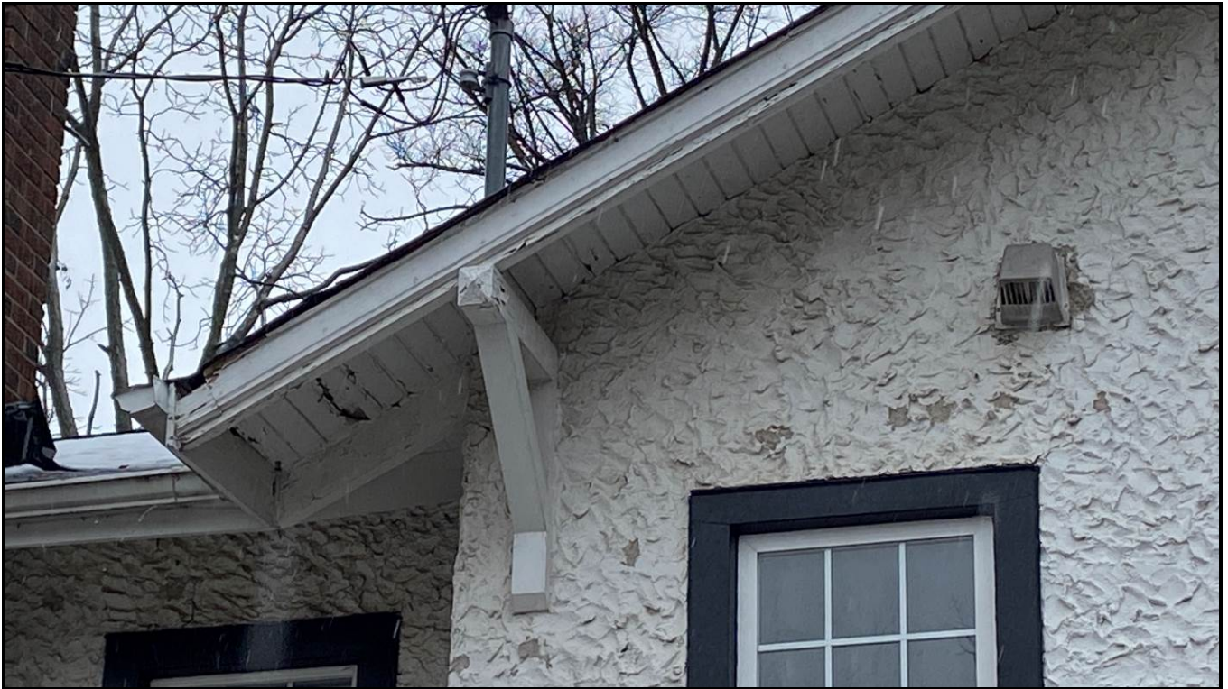
Close up of one of the wooden brackets that are spaced underneath the eaves, as well as wooden soffit and fascia. Source: Town of Oakville Planning Services Staff
