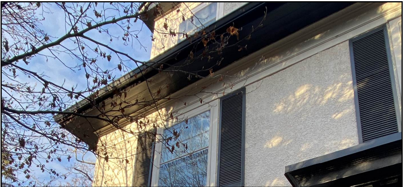
Close-up of the friezeboard and wooden soffit. Source: Town of Oakville Planning Services Staff
