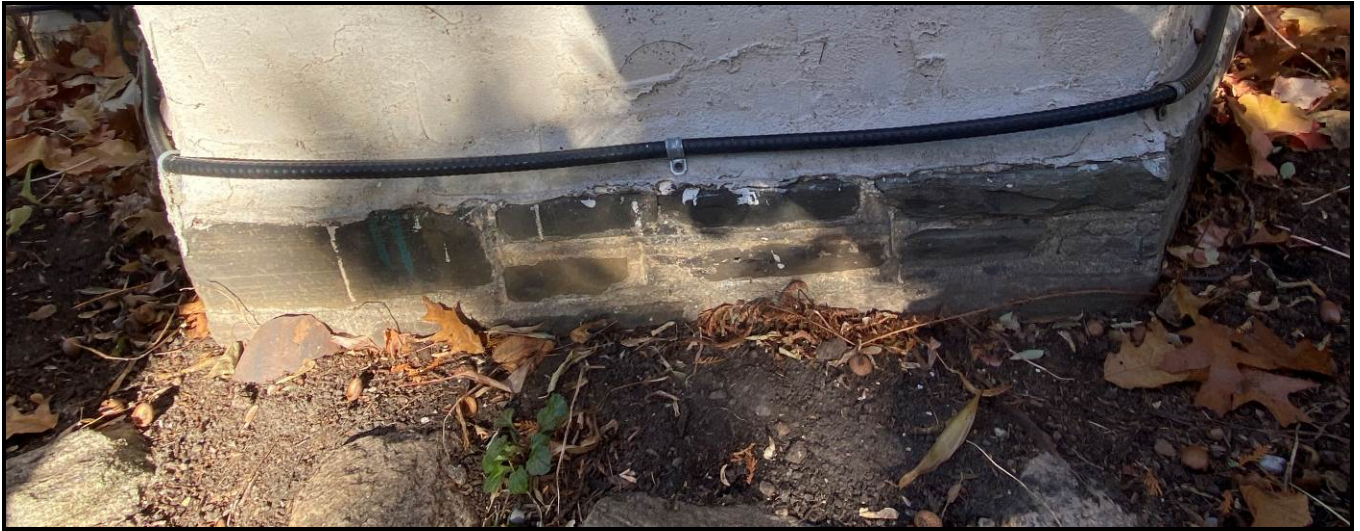
Close up of the foundation on the west elevation. Source: Town of Oakville Planning Services Staff
